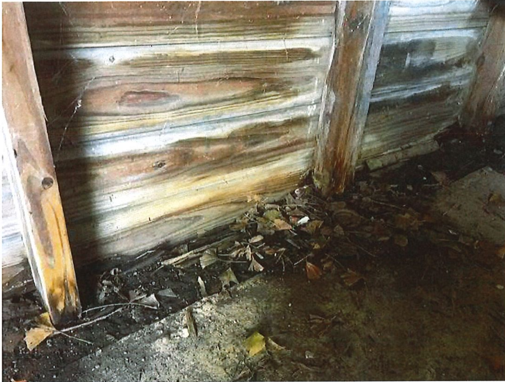
Deteriorated ends of studs
