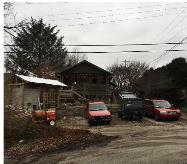
View of Alley from existing Garage Door on West side of Garage
