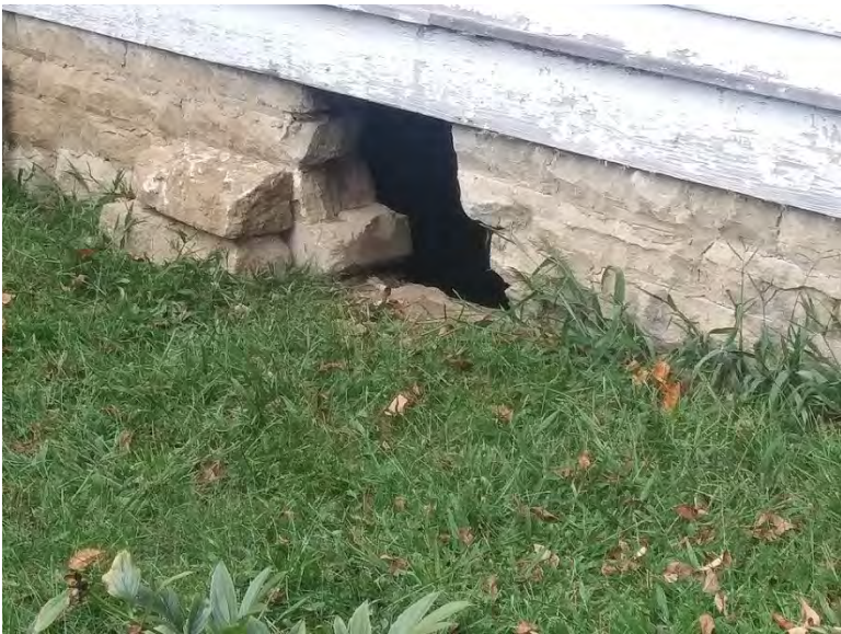
Hole in south foundation wall
