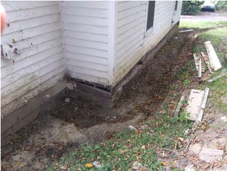
North foundation wall - Sill damage at northeast corner
