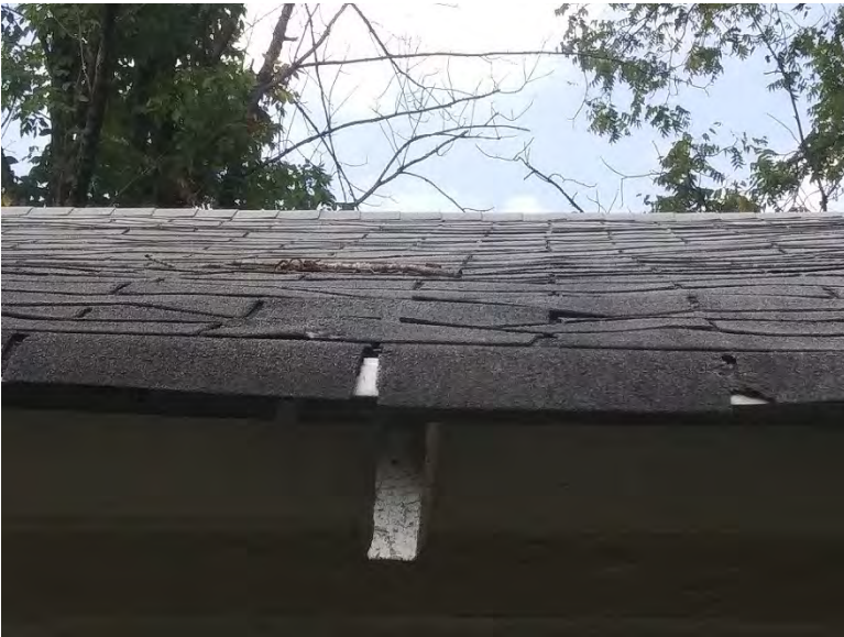
Wavy Roof Surface due to sagging rafters and poor shingles
