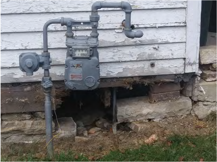
Hole in south foundation wall
