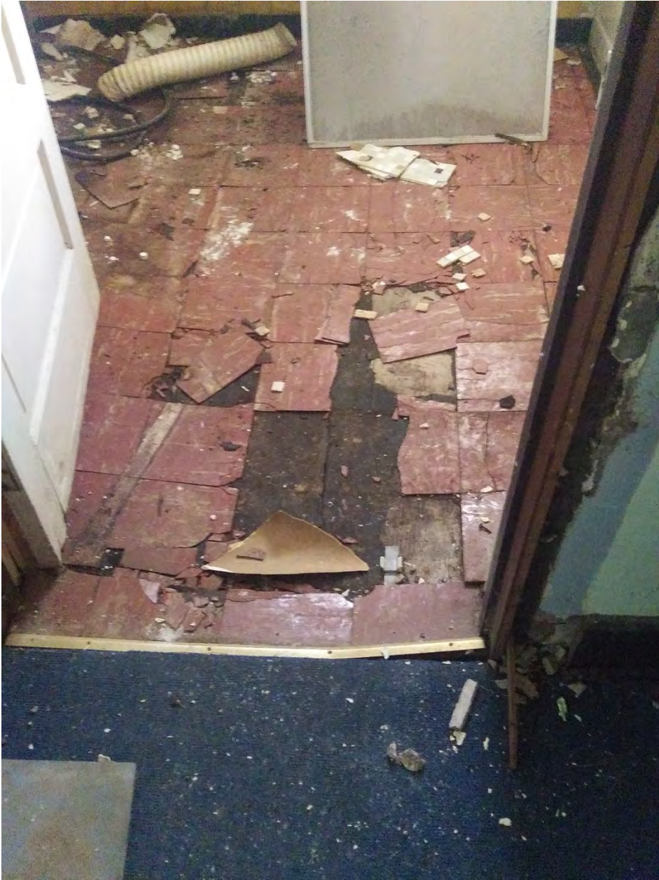
Bathroom floor water damage
