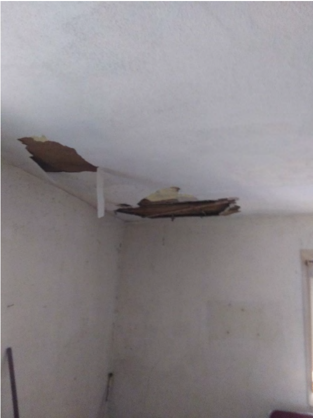
Water damage at southeast corner
