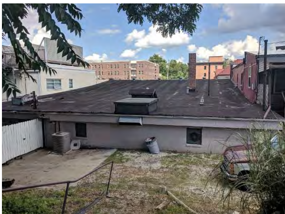
West Façade (roof sagging & failing)
