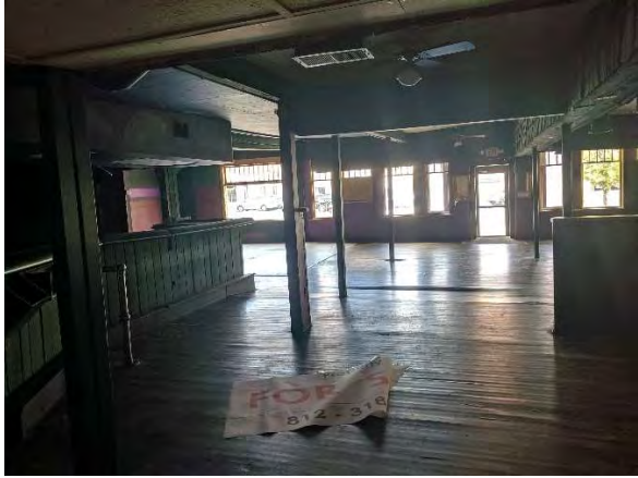
North Building looking east (sinking columns)
