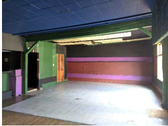
North Building looking north (sagging beam)
