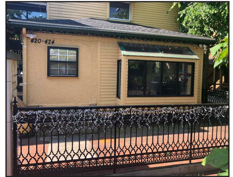
Incompatible: Enclosed Porch
