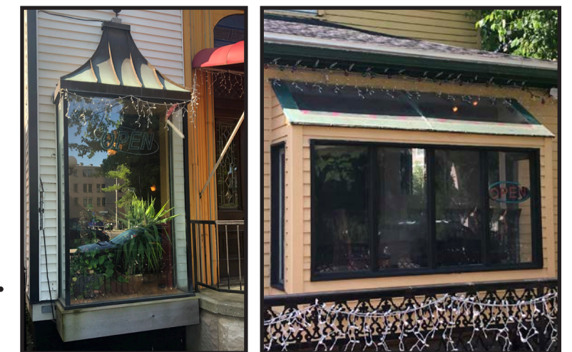
Examples of Incompatible Windows
