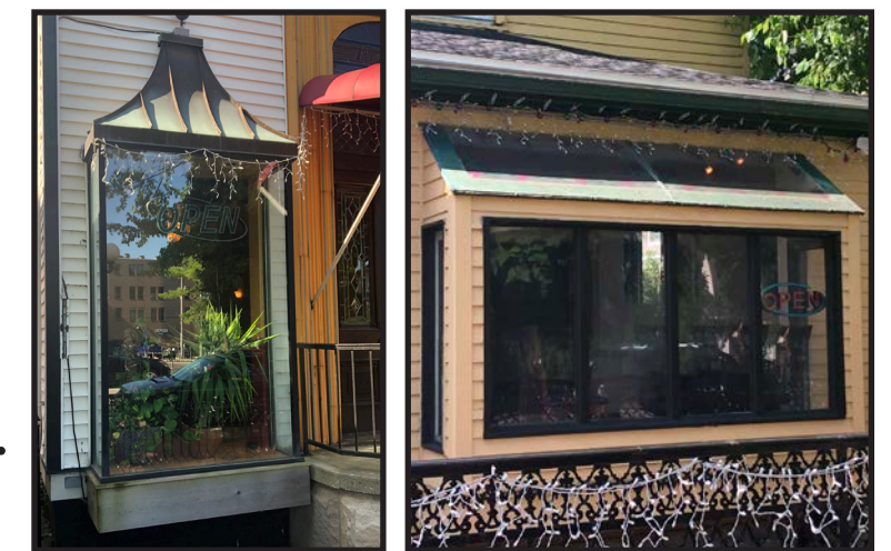
Examples of Incompatible Windows
