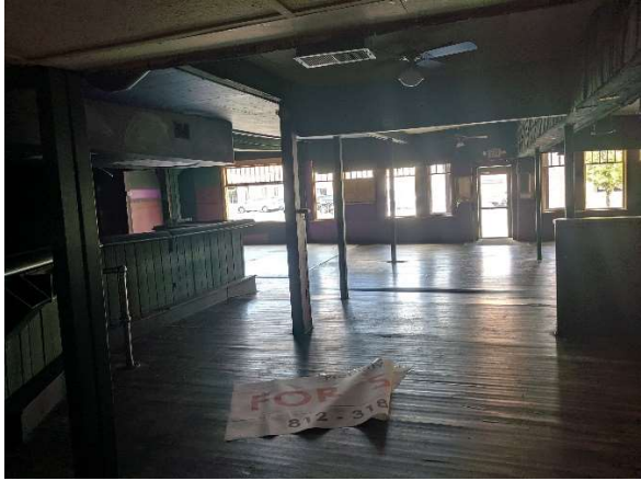
North Building looking east (sinking columns)
