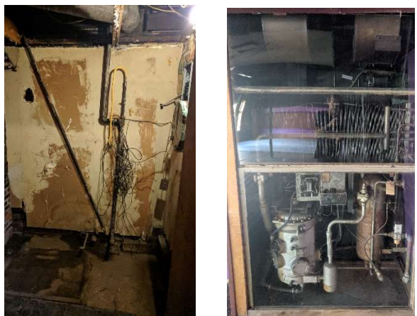
South Building utilities (exposed wiring & mech)
