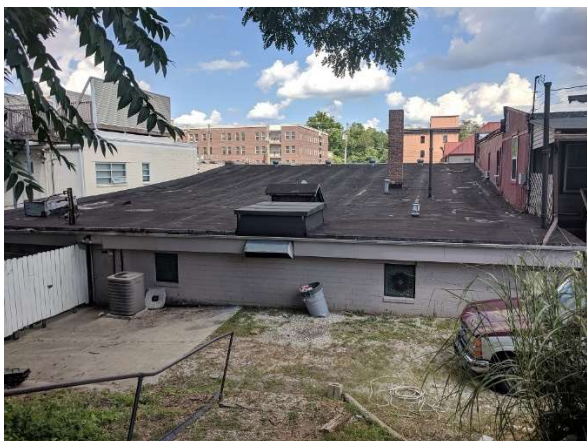
West Façade (roof sagging & failing)
