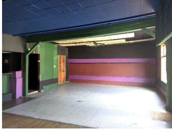
North Building looking north (sagging beam)
