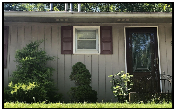
Not Recommended: Vertically-oriented siding.
