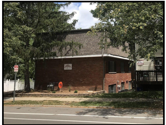
Not Recommended: Entry door missing from street facing side.
