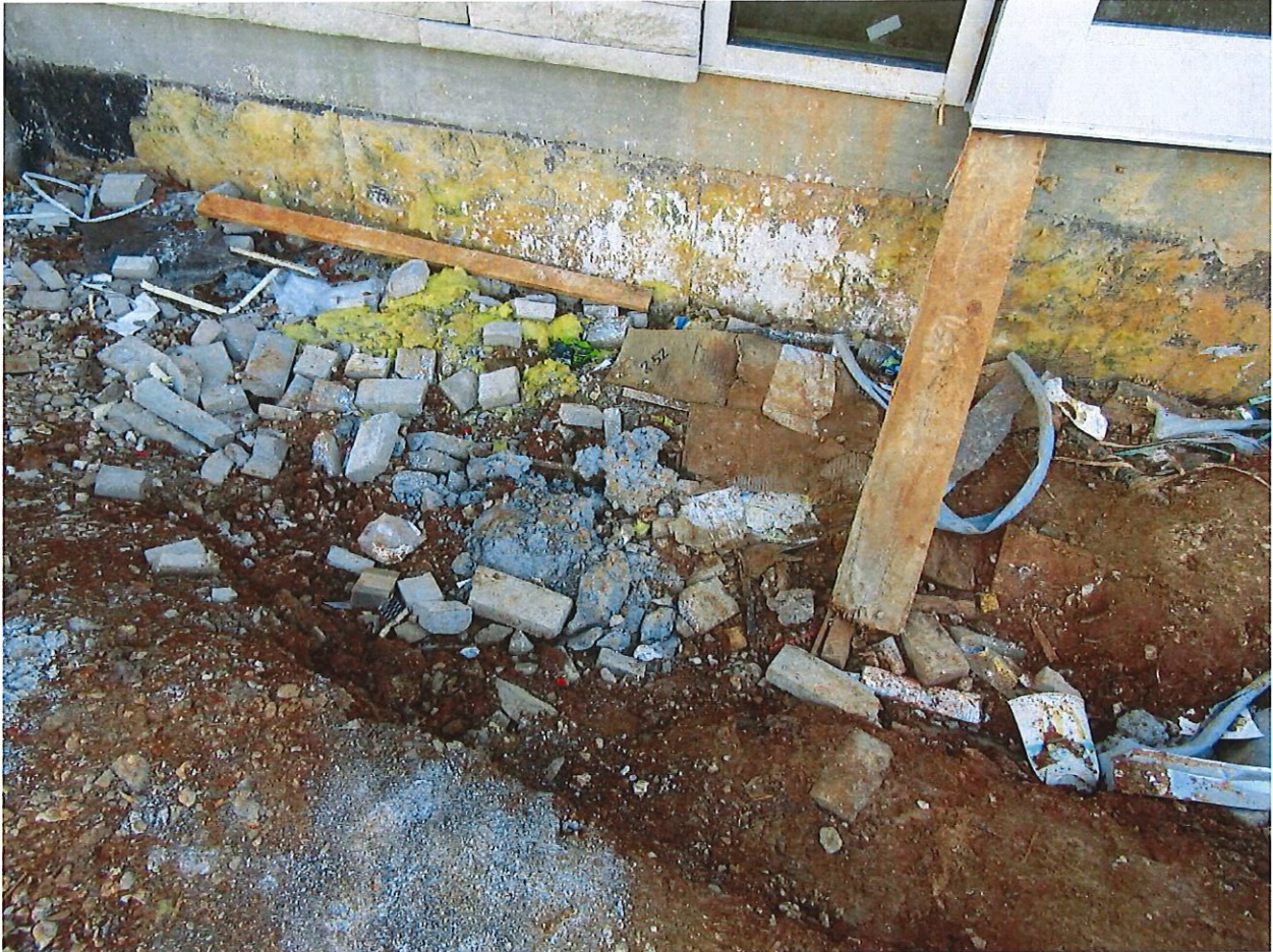
Figure 1: Improperly disposed of materials.
