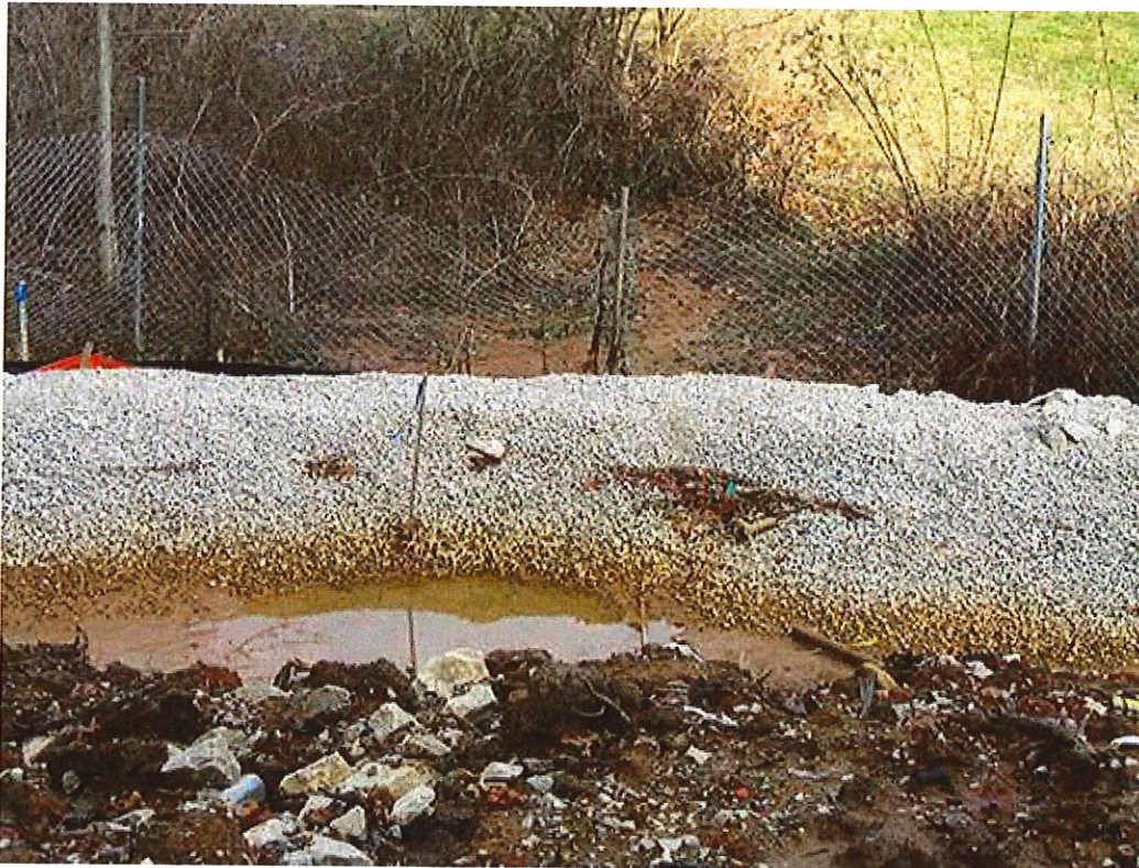
Figure 22: The upper basin of the structure is full of sediment and not working effectively.
