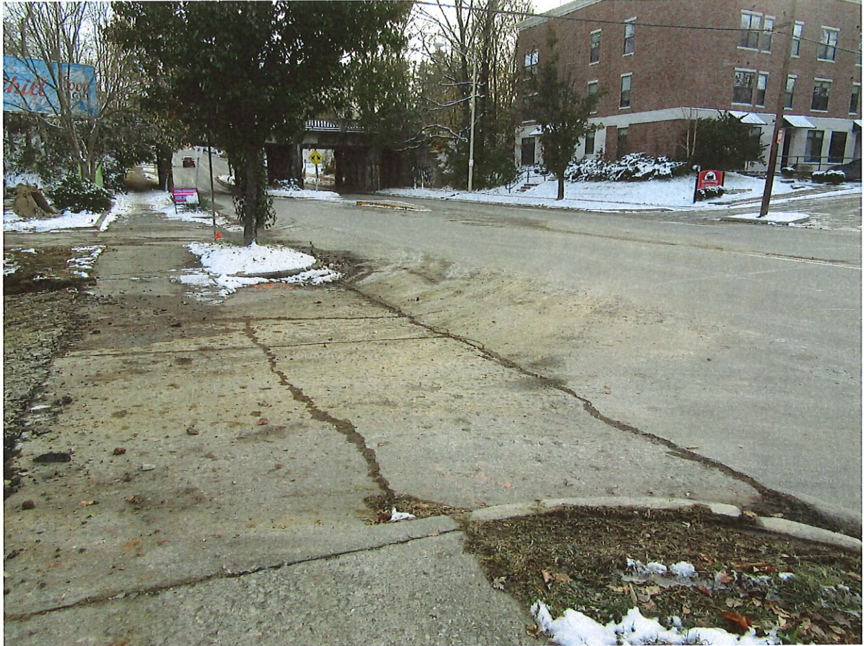
Figure 5: Sediment tracking, College Avenue.
