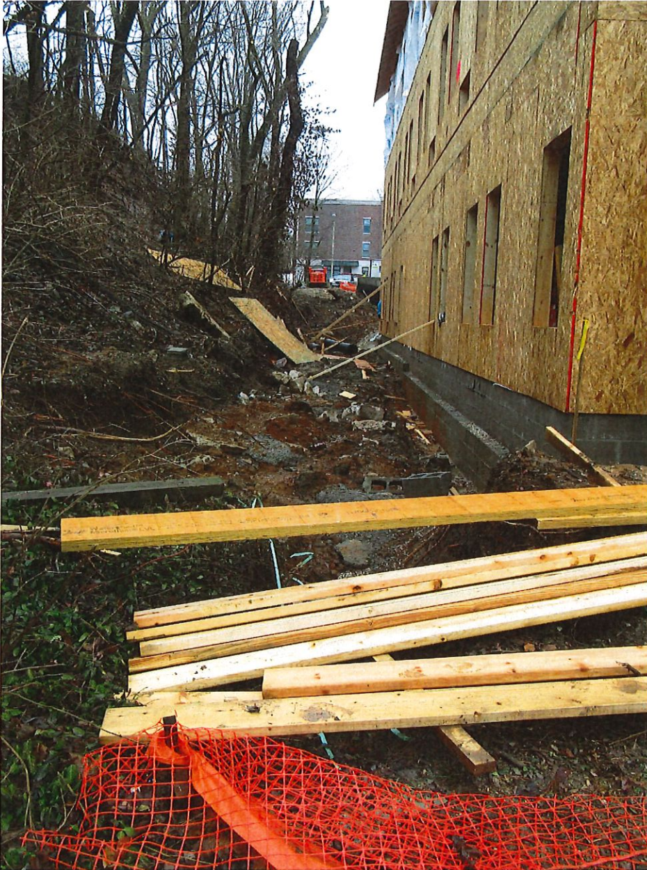
Figure 7: Improperly disposed of construction materials.
