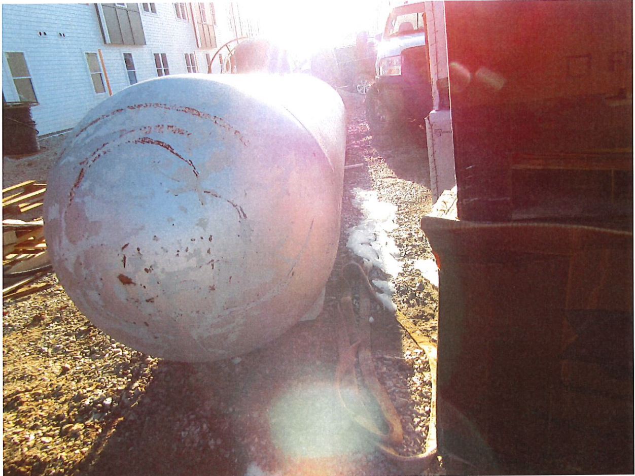
Figure 11: Gas tank on site was not labeled.
