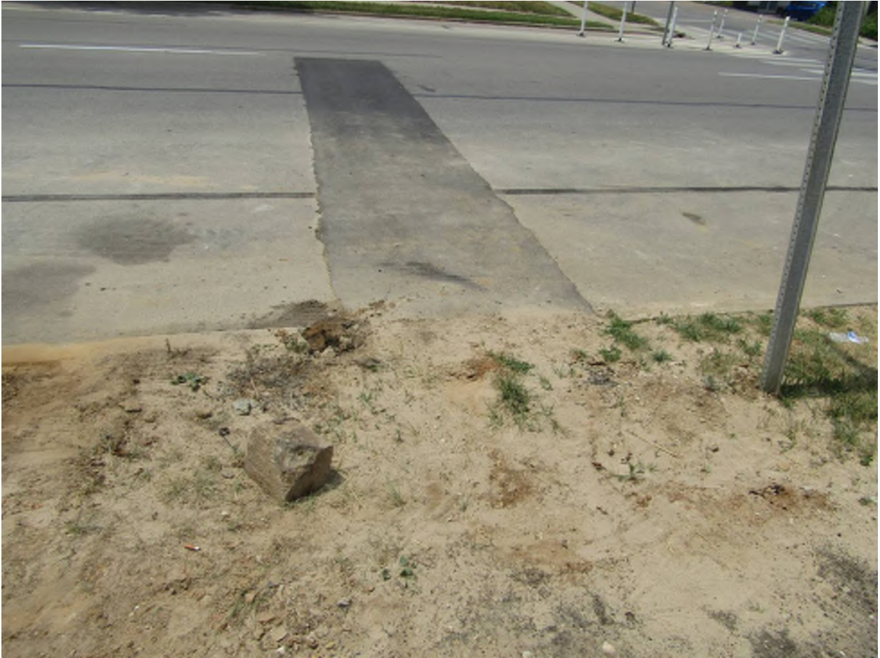
Figure 3: Sediment in the tree plot along N. College Ave.
