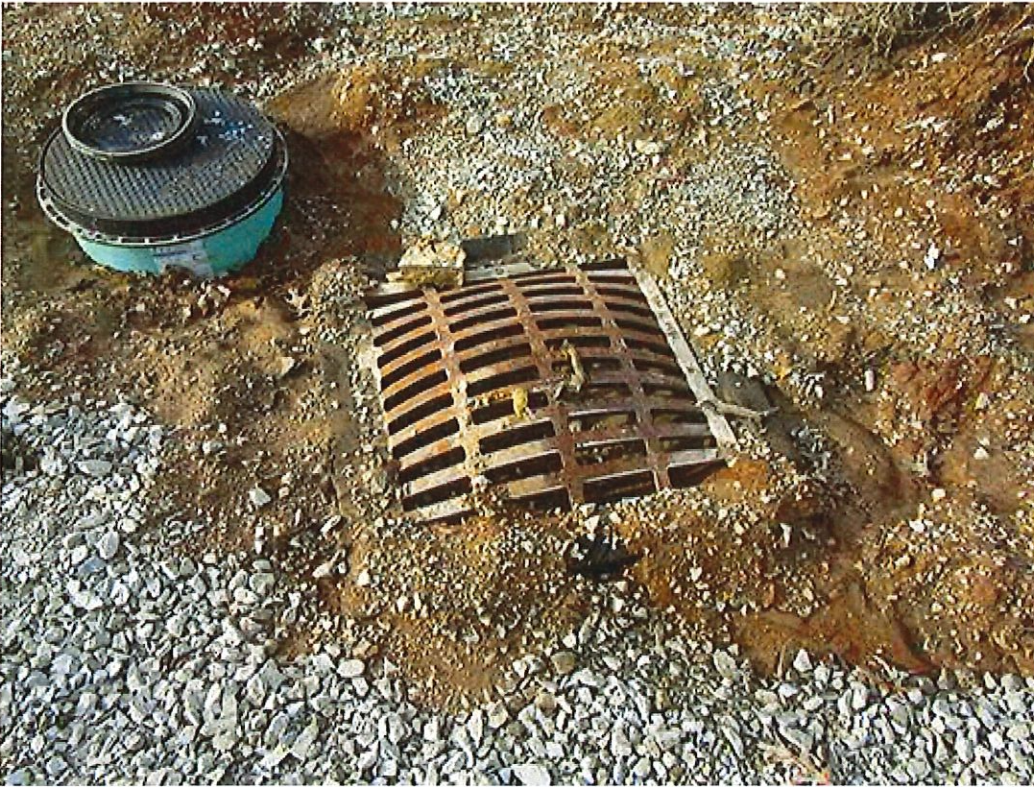
Figure 17: Filter fabric is in place, but needs maintenance.
