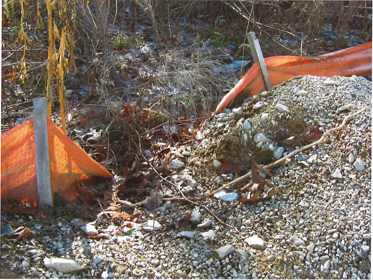
Figure 8: Failed section of silt fence needs to be repaired or replaced.
