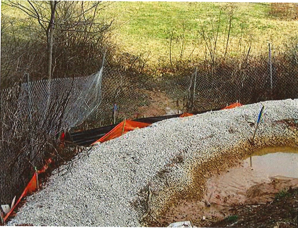
Figure 21: This measure to control sediment is not working; sediment has flowed through it and onto nearby vegetation/property.
