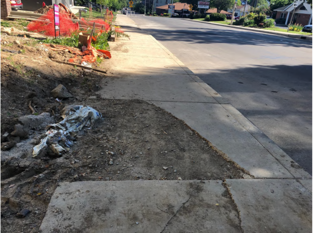
Figure 9: Damaged sidewalk panel along Walnut Street.
