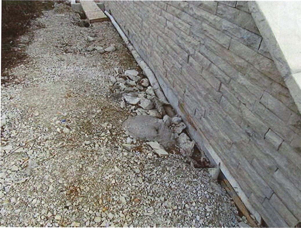
Figure 9: Inappropriately disposed of construction material.
