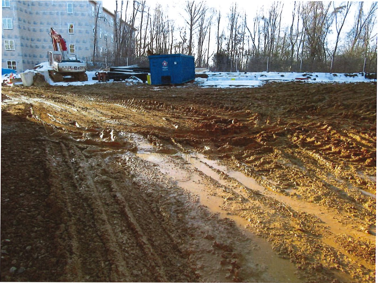
Figure 4: Muddy access drive and parking area.
