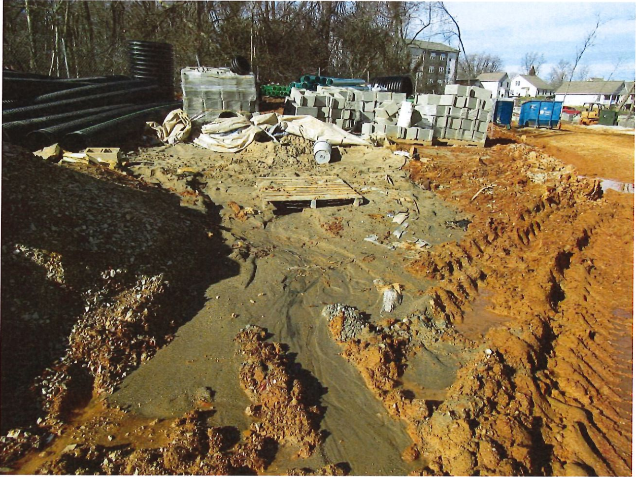
Figure 2: Improperly disposed of materials.
