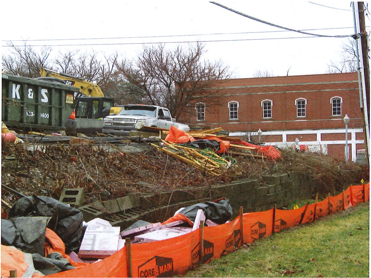
Figure 4: Improperly disposed of construction materials.
