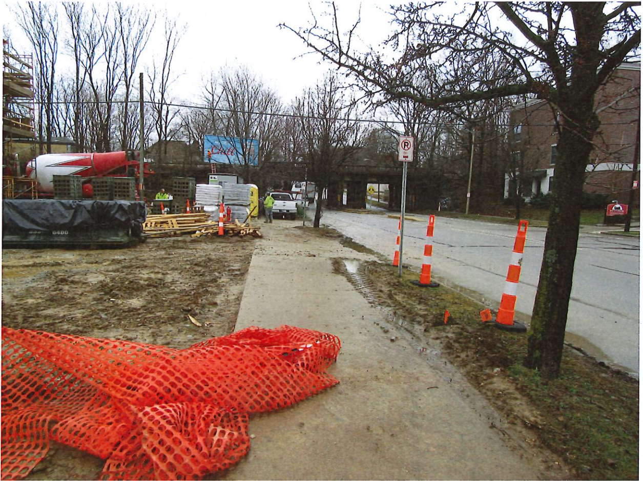
Figure 8: Construction drive is muddy and causing tracking out onto College.
