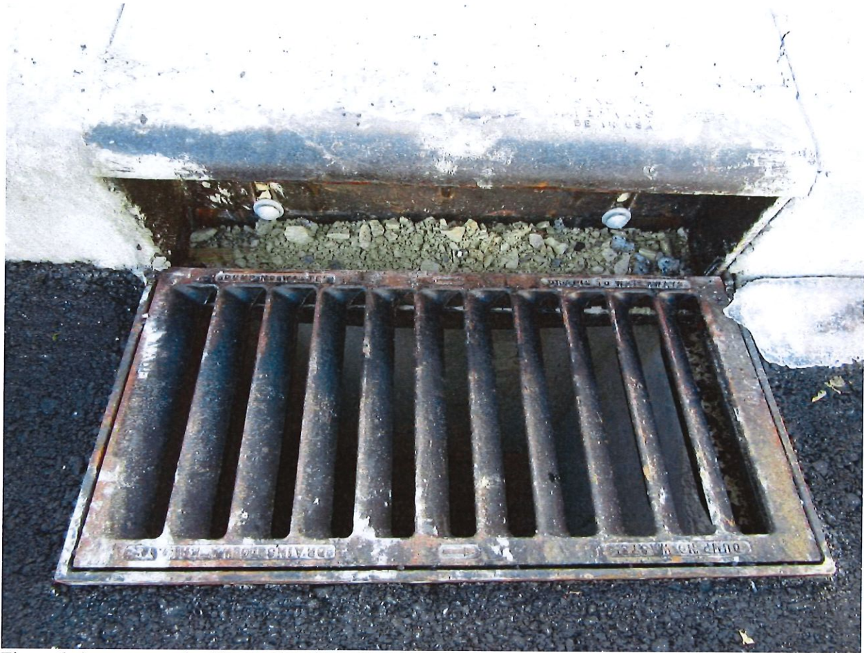
Figure 6: Aggregate and evidence of concrete disposed of in a storm inlet.
