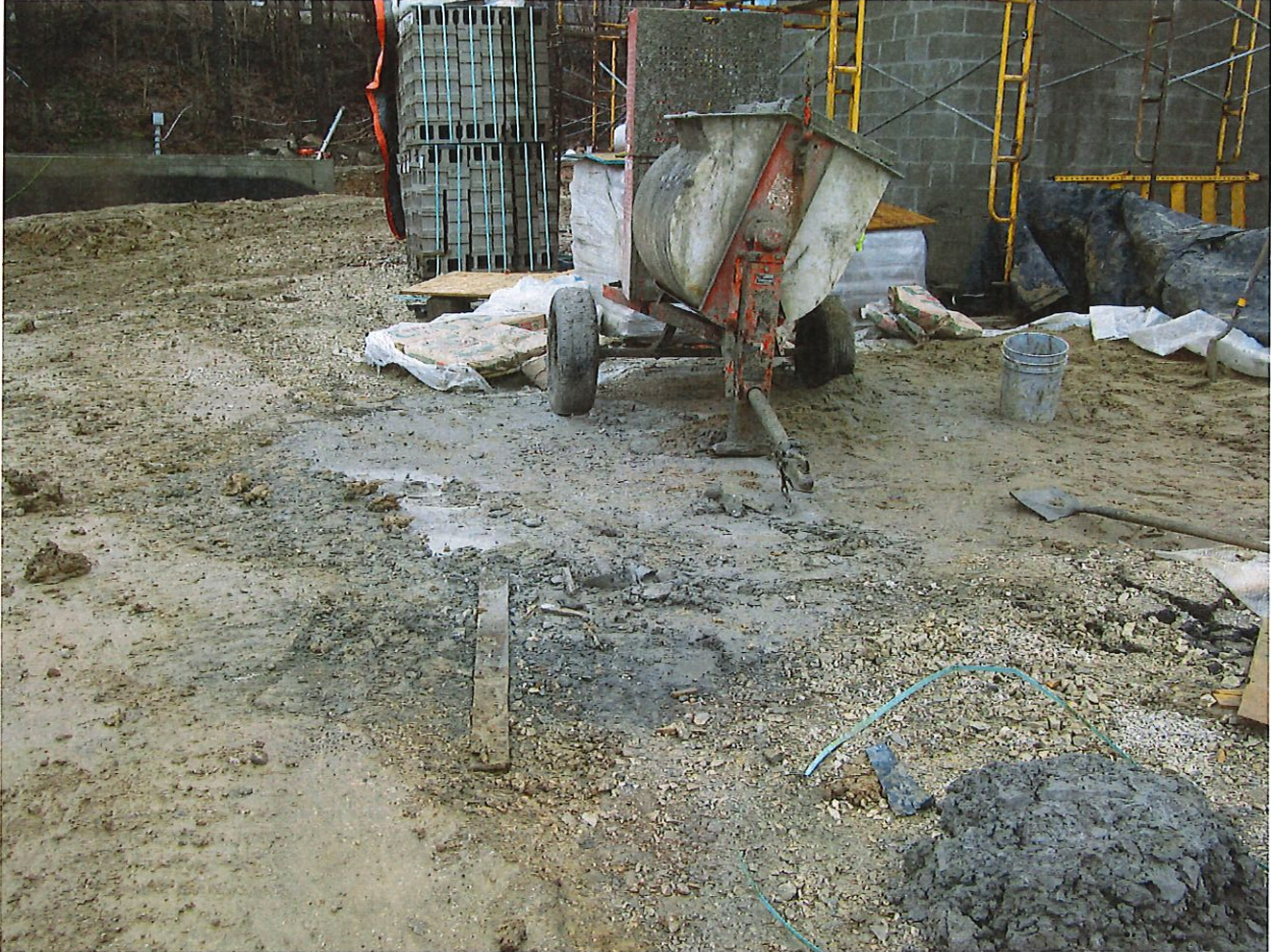
Figure 3: Improperly contained/disposed of construction materials.
