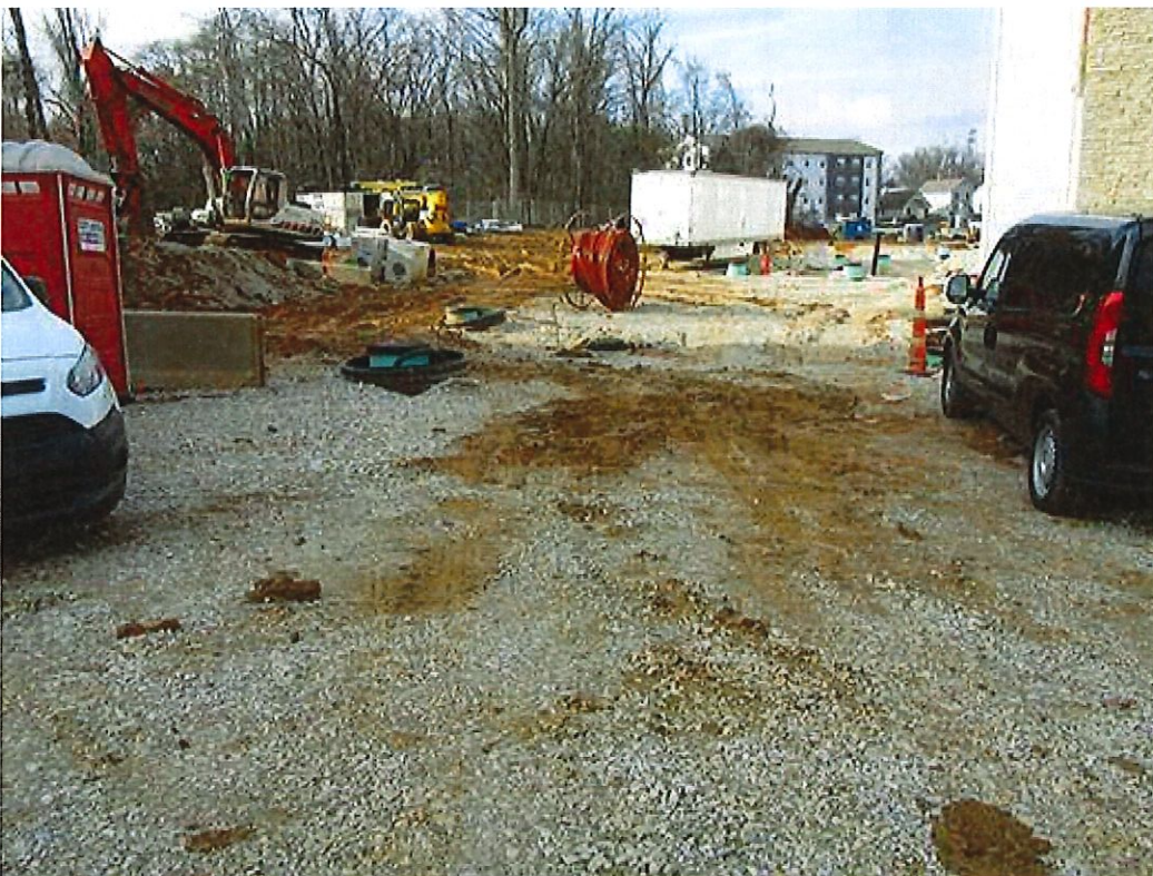
Figure 6: Muddy parking area and drive.
