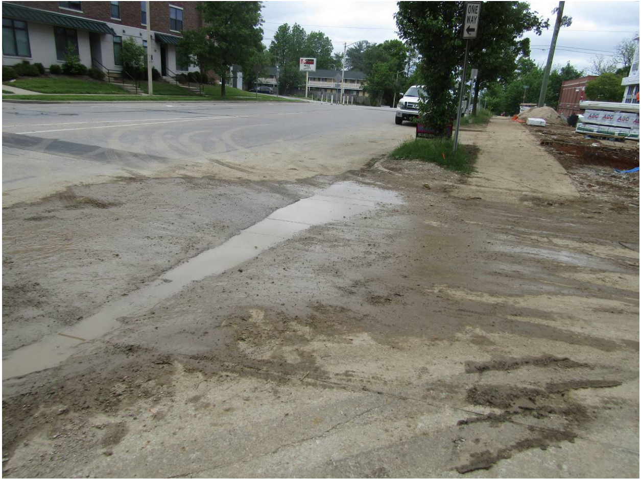
Figure 1: Tracking of sediment onto N. College Ave.
