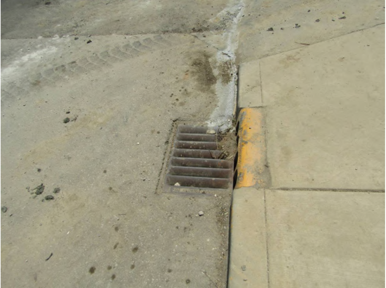
Figure 6: Tracking and concrete going into N. Walnut St inlet without protection.
