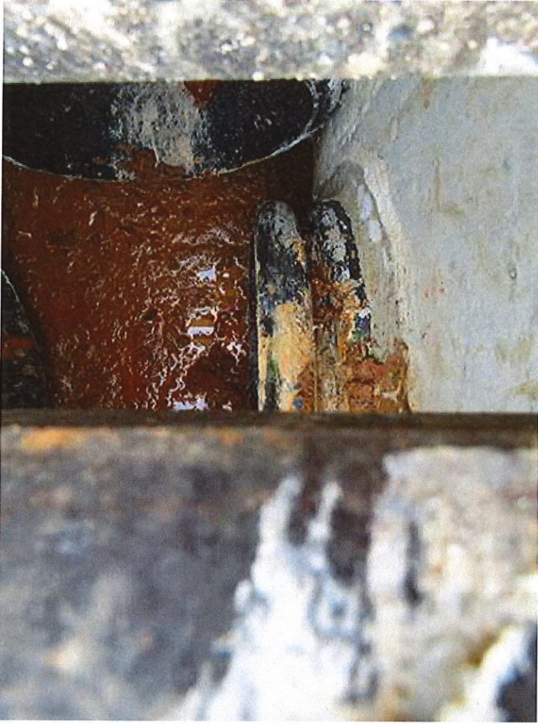
Figure 18: Sediment inside a storm inlet.
