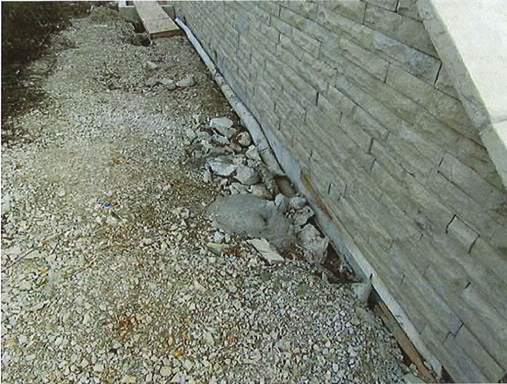
Figure 9: Inappropriately disposed of construction material.
