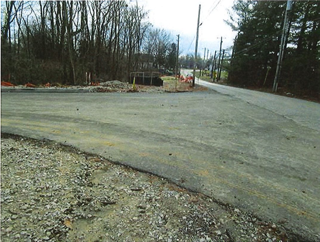
Figure 1: Tracking of sediment onto Crescent Drive.
