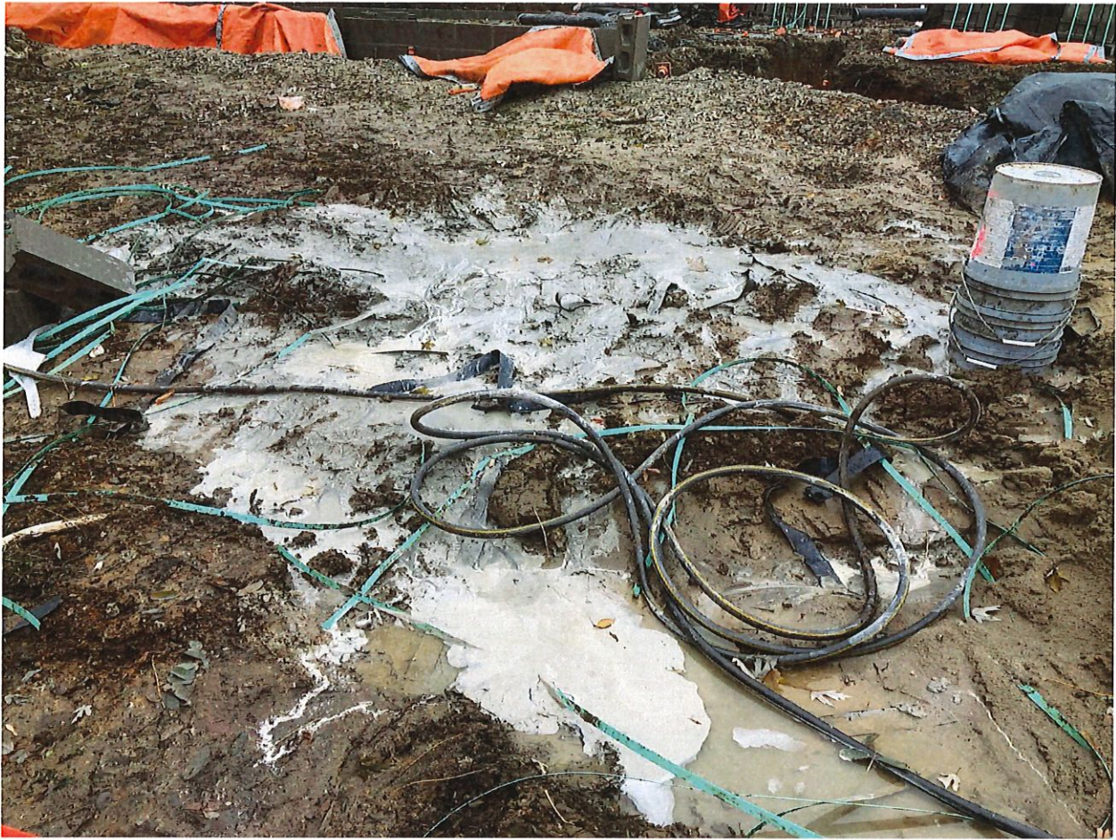
Figure 1: Improperly disposed of construction materials.
