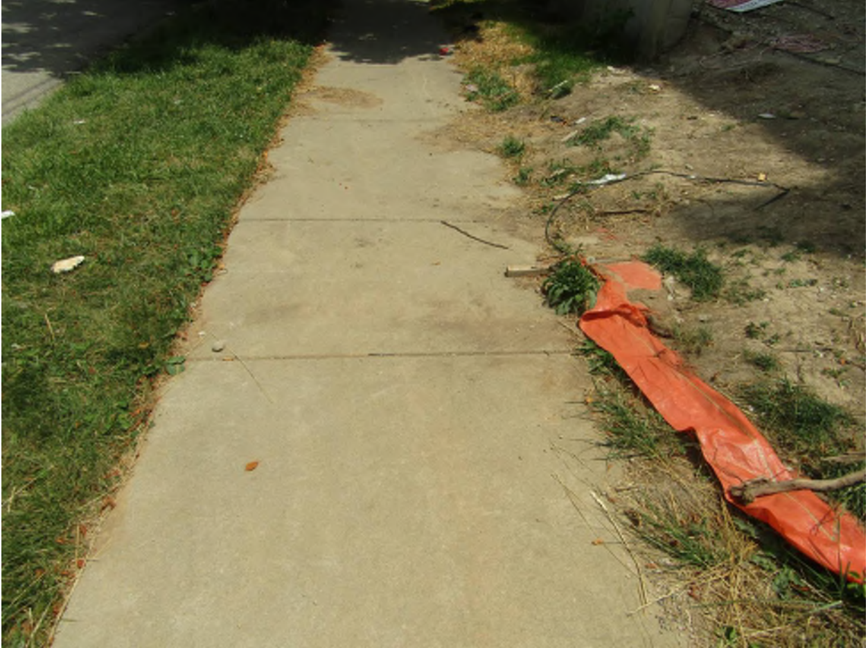
Figure 5: Silt fence collapsed into 14 th Street sidewalk.
