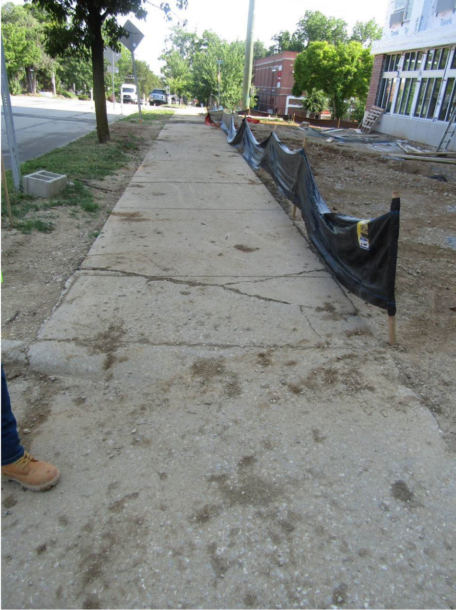
Figure 6: 7/6/2020 - Silt fence improperly installed along College Avenue.
