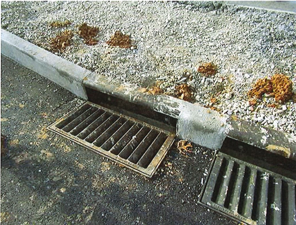
Figure 19: Unprotected storm inlets.
