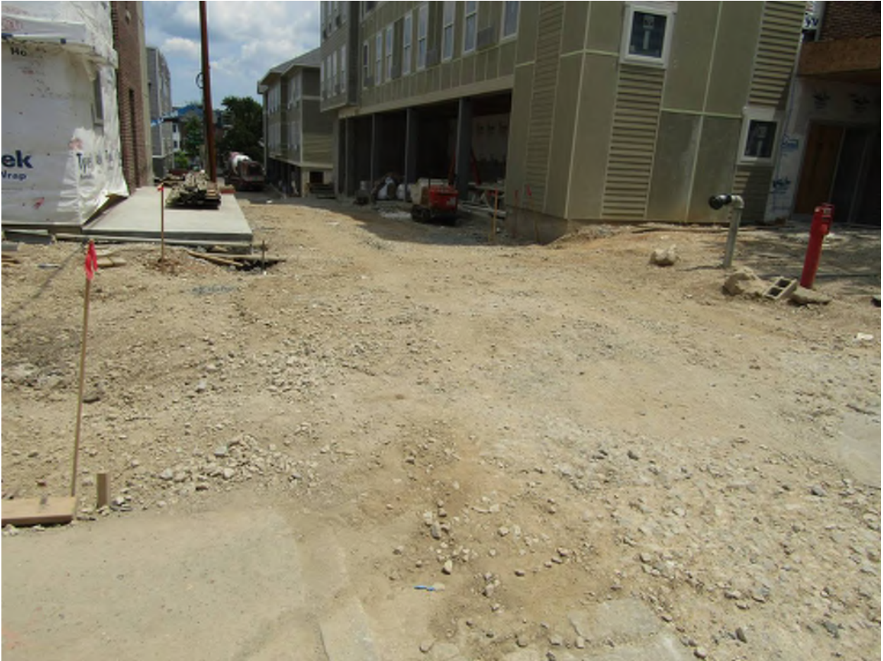
Figure 8: Construction entrance not being maintained with clean crushed stone.
