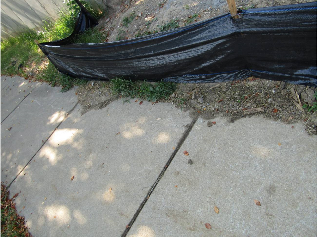
Figure 9: 7/6/2020 - Silt fence along 14 th Street not properly installed, not containing sediment to the site.
