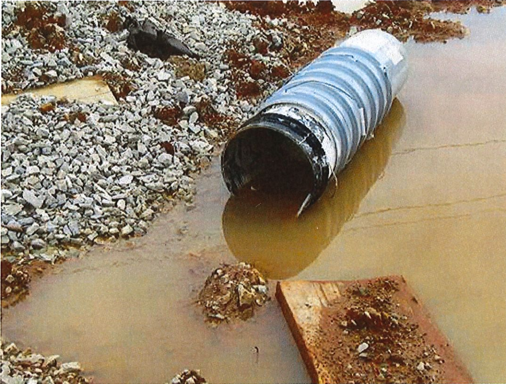
Figure 11: Inappropriately disposed of construction materials.
