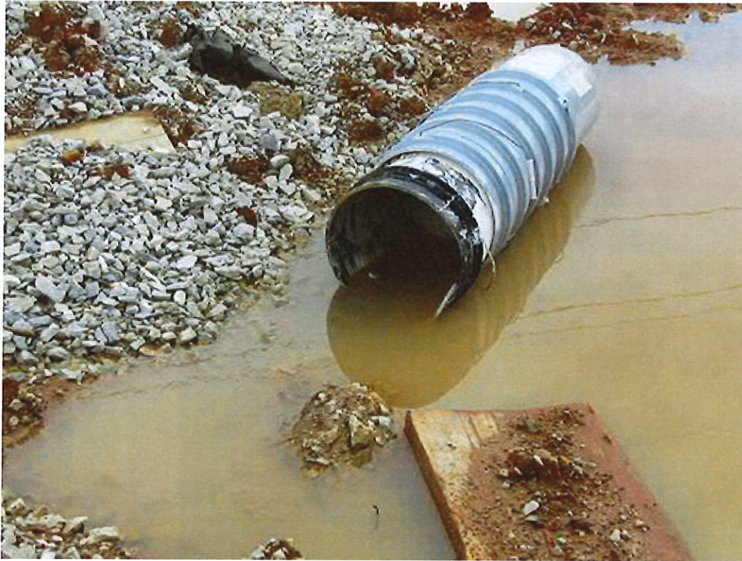
Figure 11: Inappropriately disposed of construction materials.
