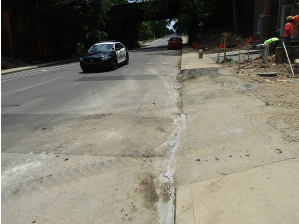
Figure 7: Concrete debris tracked into N. Walnut Street.
