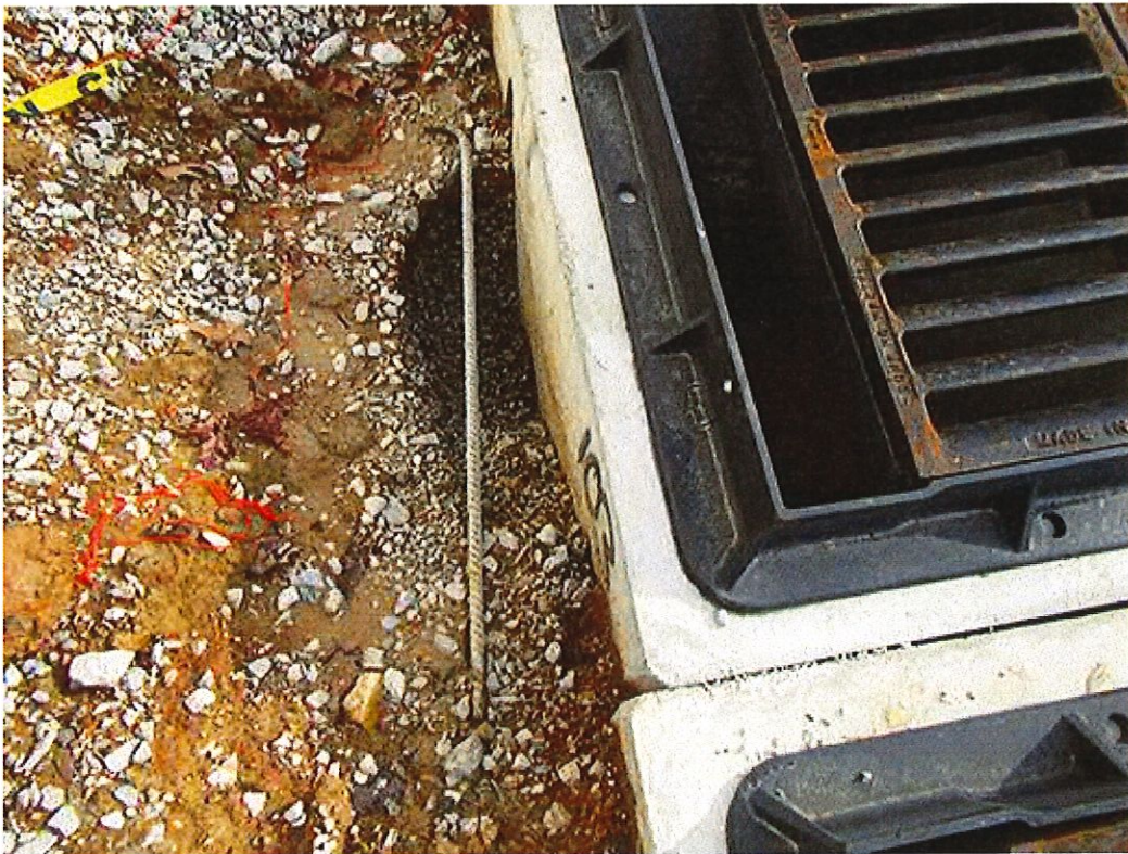
Figure 16: Sediment erosion around the storm inlet is causing sediment to flow directly into the inlet.
