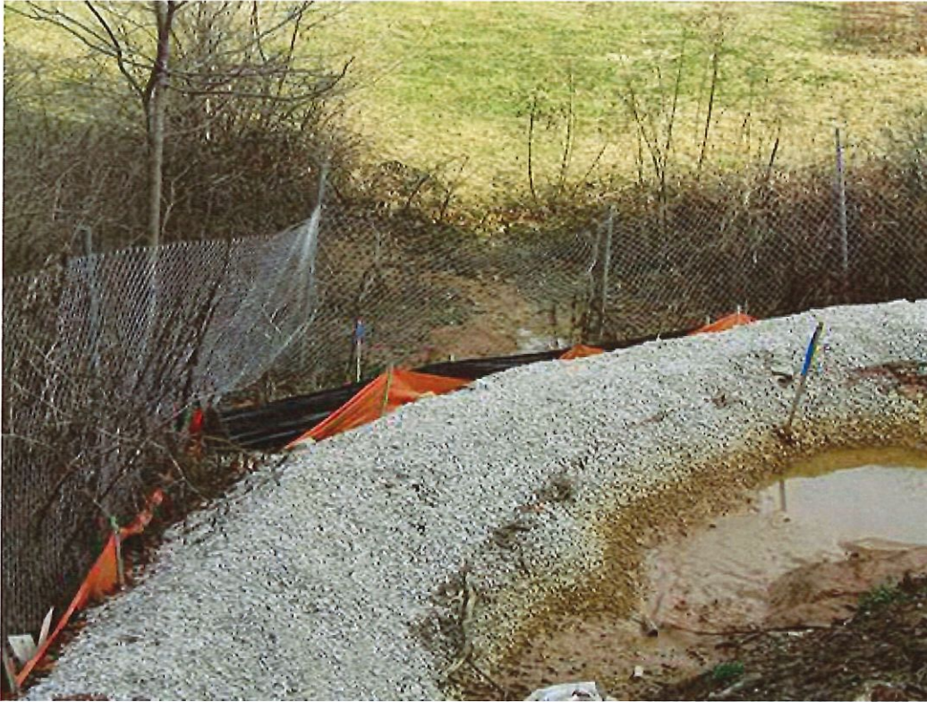
Figure 21: This measure to control sediment is not working; sediment has flowed through it and onto nearby vegetation/property.
