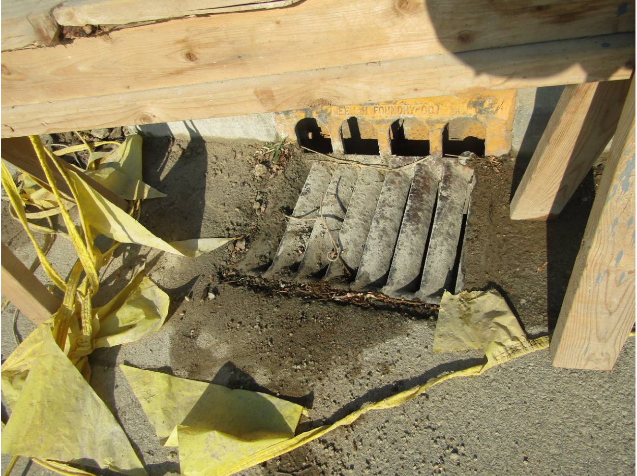
Figure 1:7/6/2020 - Inlet north of the alley along Walnut Street not protected and with sediment/unknown substance flowing into it.
