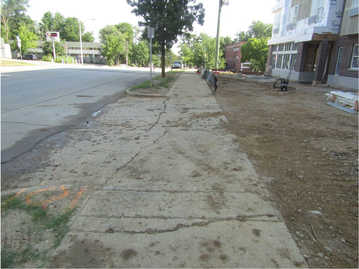
Figure 5: 7/6/2020 - Sediment tracked into sidewalk and into the street. This area of the site has been exposed for longer than 14 days.
