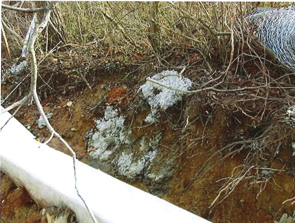
Figure 12: Inappropriately disposed of construction materials.
