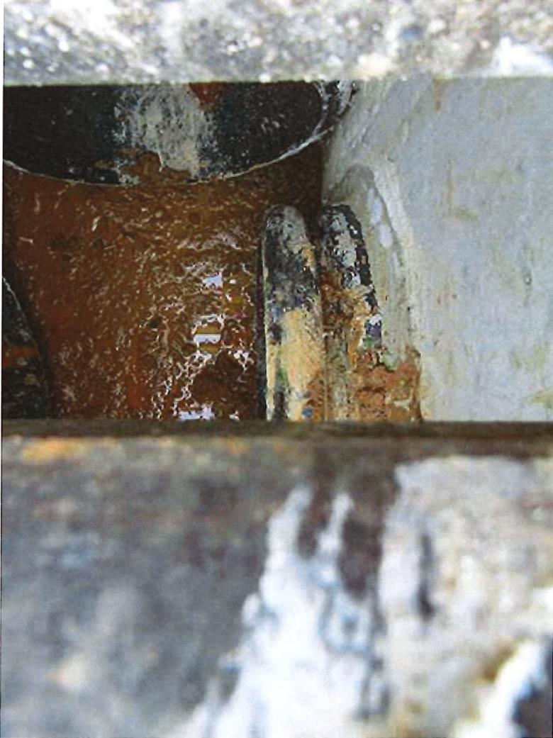
Figure 18: Sediment inside a storm inlet.
