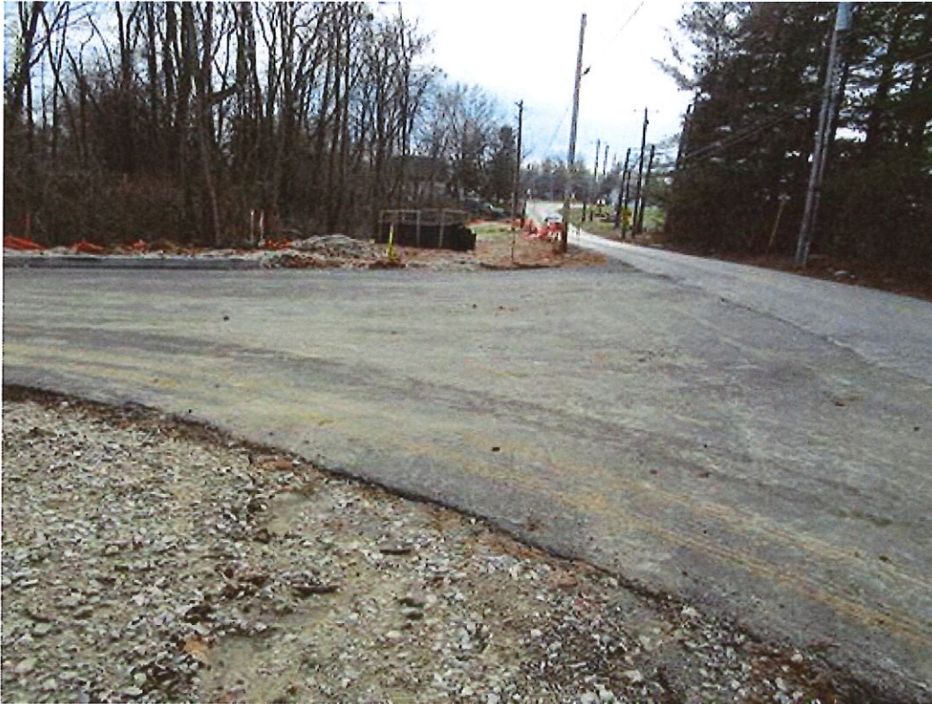
Figure 1: Tracking of sediment onto Crescent Drive.
