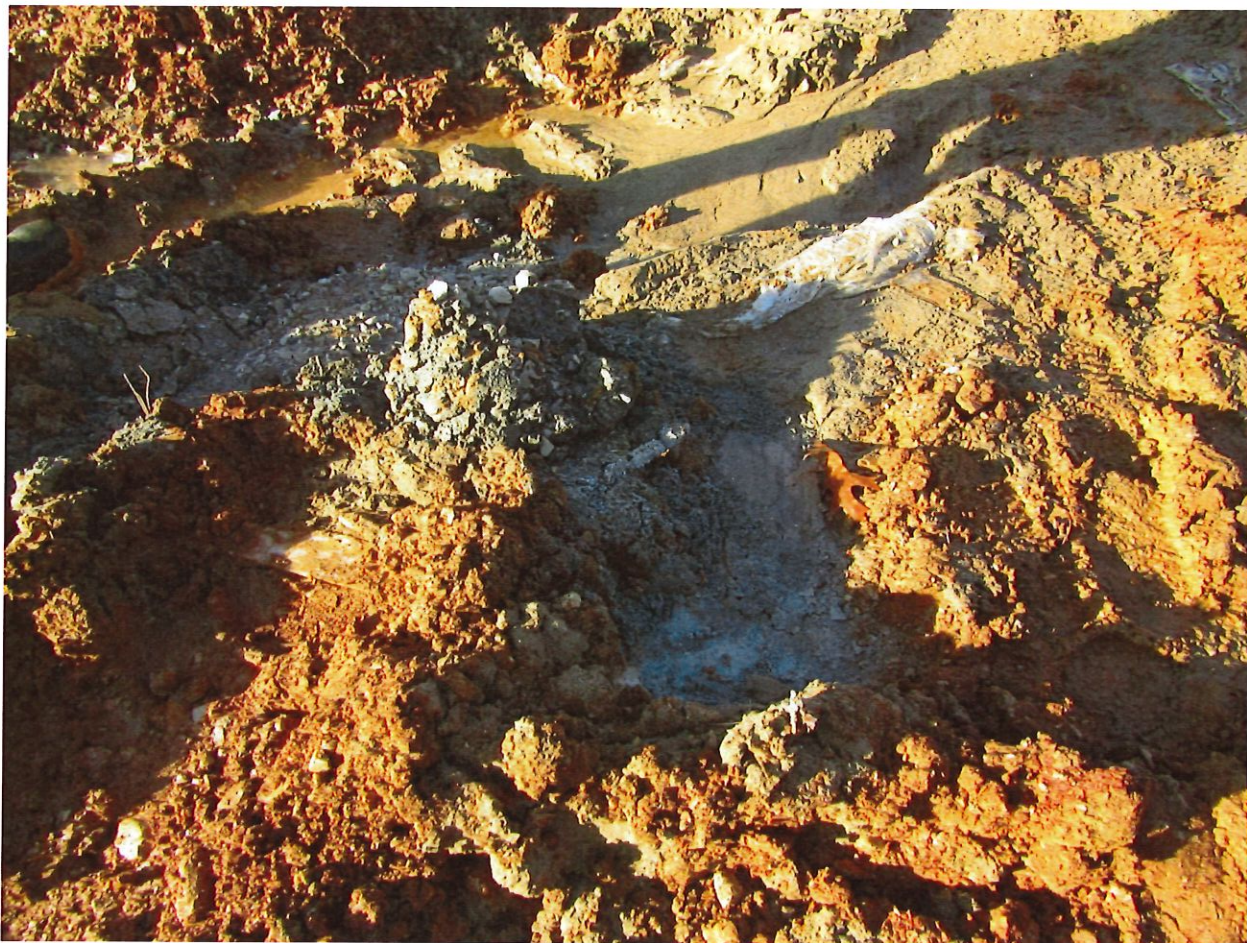
Figure 10: Concrete washed out onto the ground.
