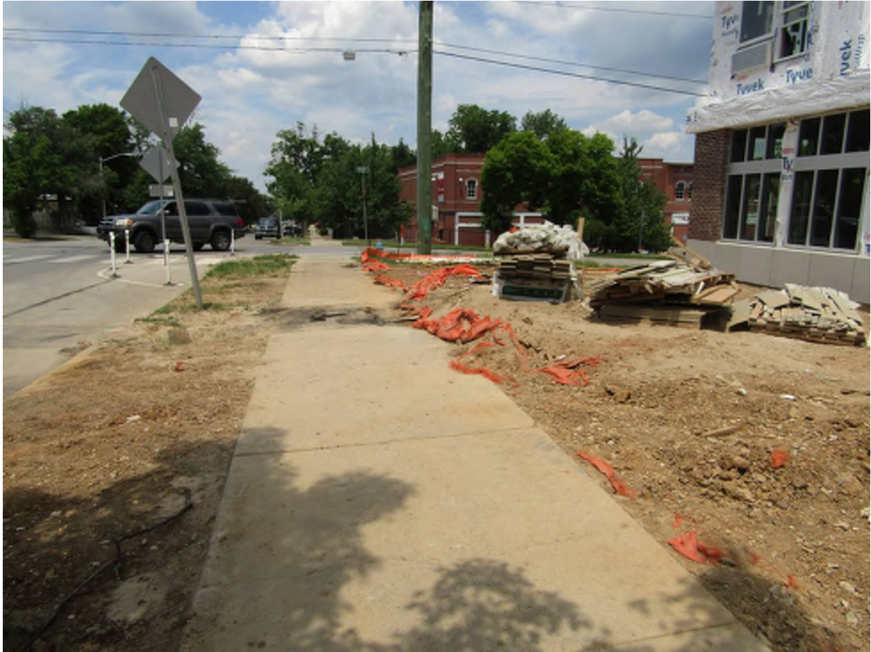
Figure 2: Silt fence collapsed along N. College Ave.
