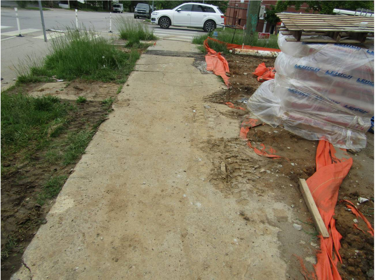
Figure 4: Silt fence collapsed and sediment tracked onto sidewalk.
