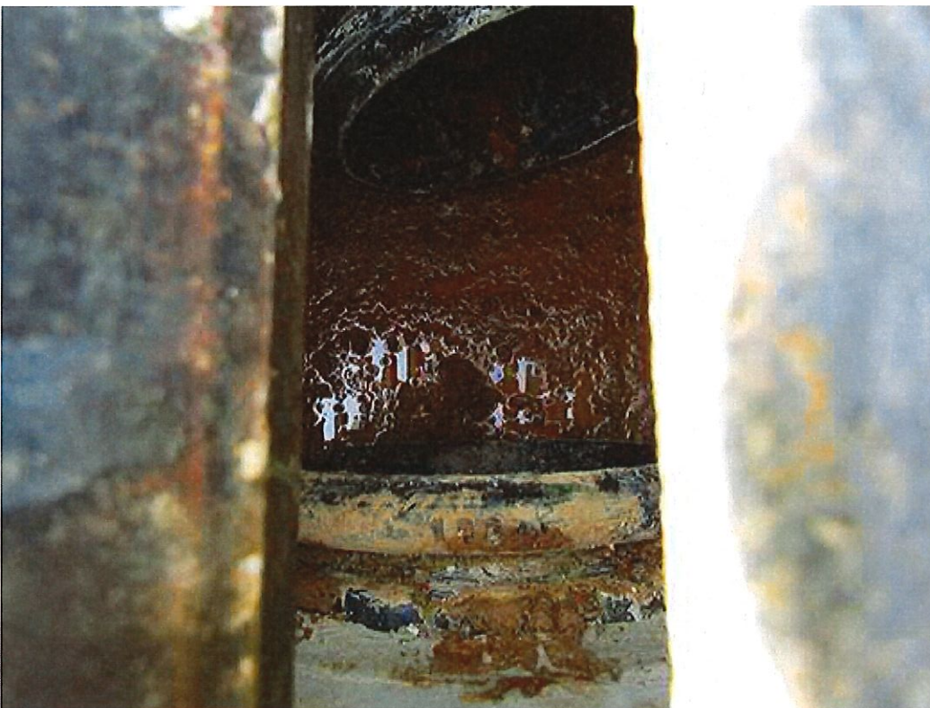
Figure 20: Sediment inside a storm inlet.
