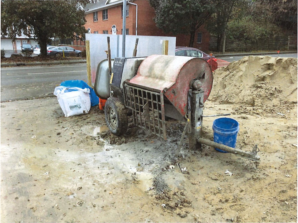
Figure 2: Improperly disposed of construction materials.
