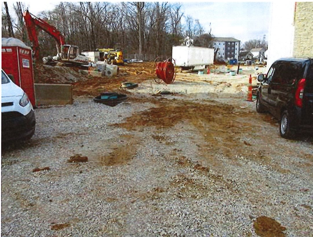
Figure 6: Muddy parking area and drive.
