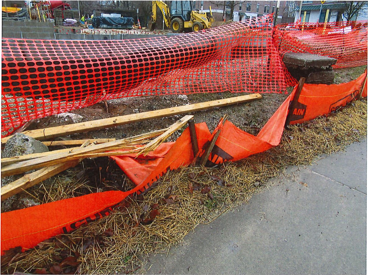
Figure 1: Improperly installed silt fence.
