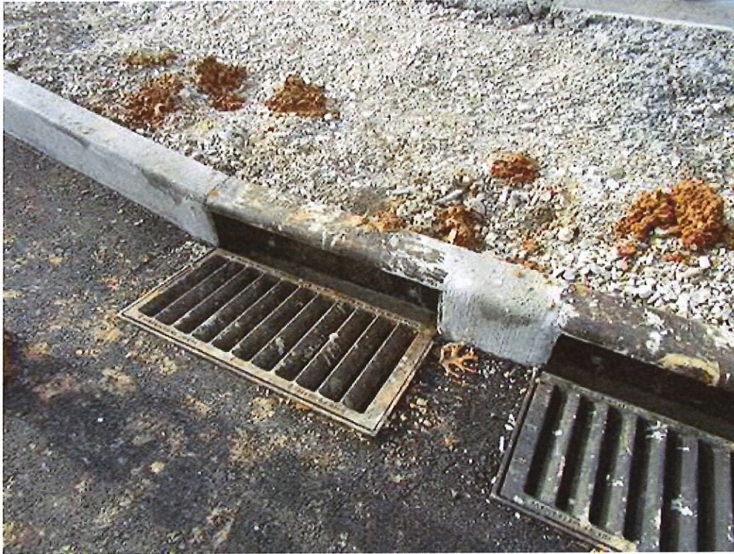
Figure 19: Unprotected storm inlets.
