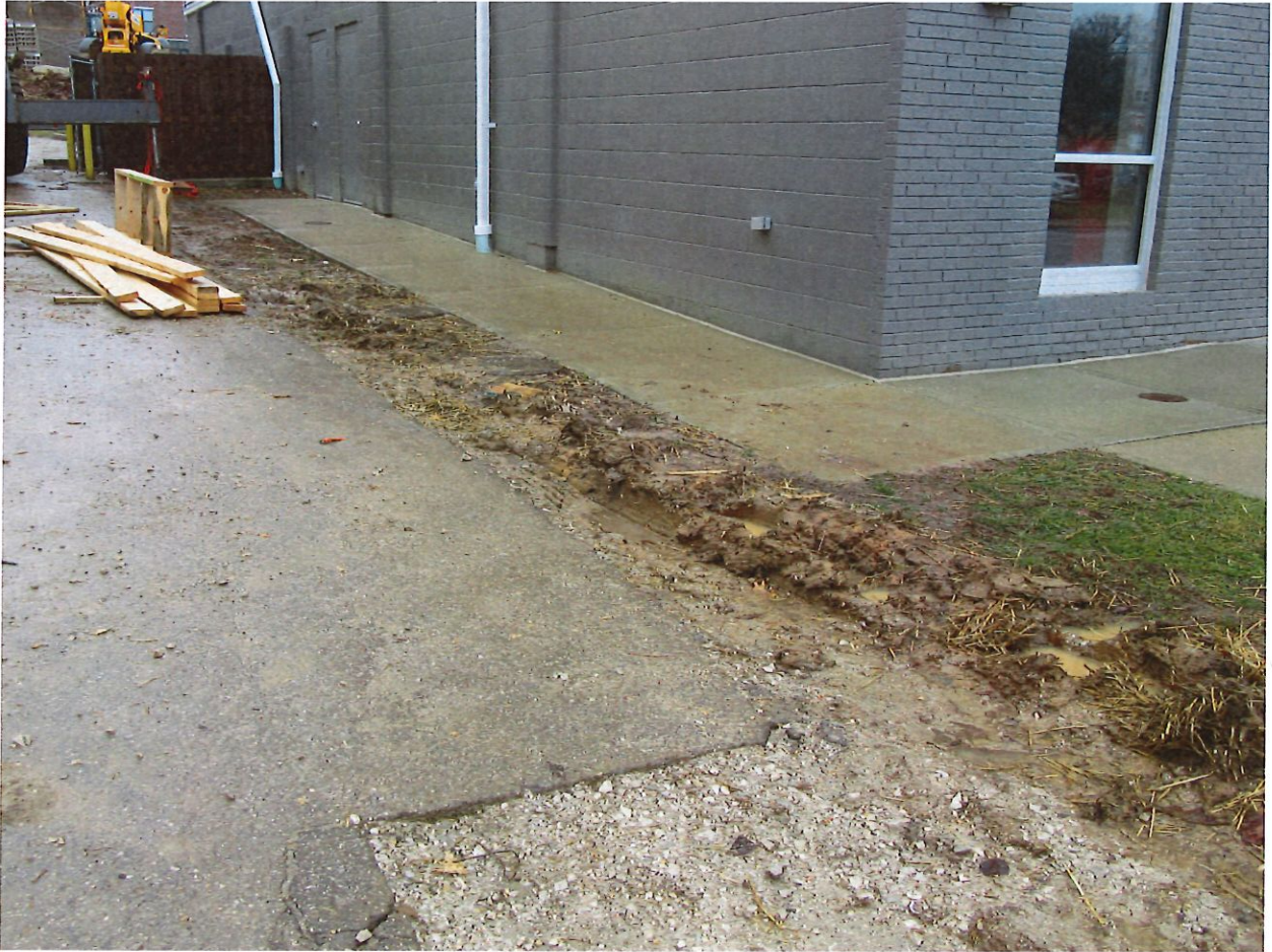
Figure 6: Disturbed area not properly stabilized.
