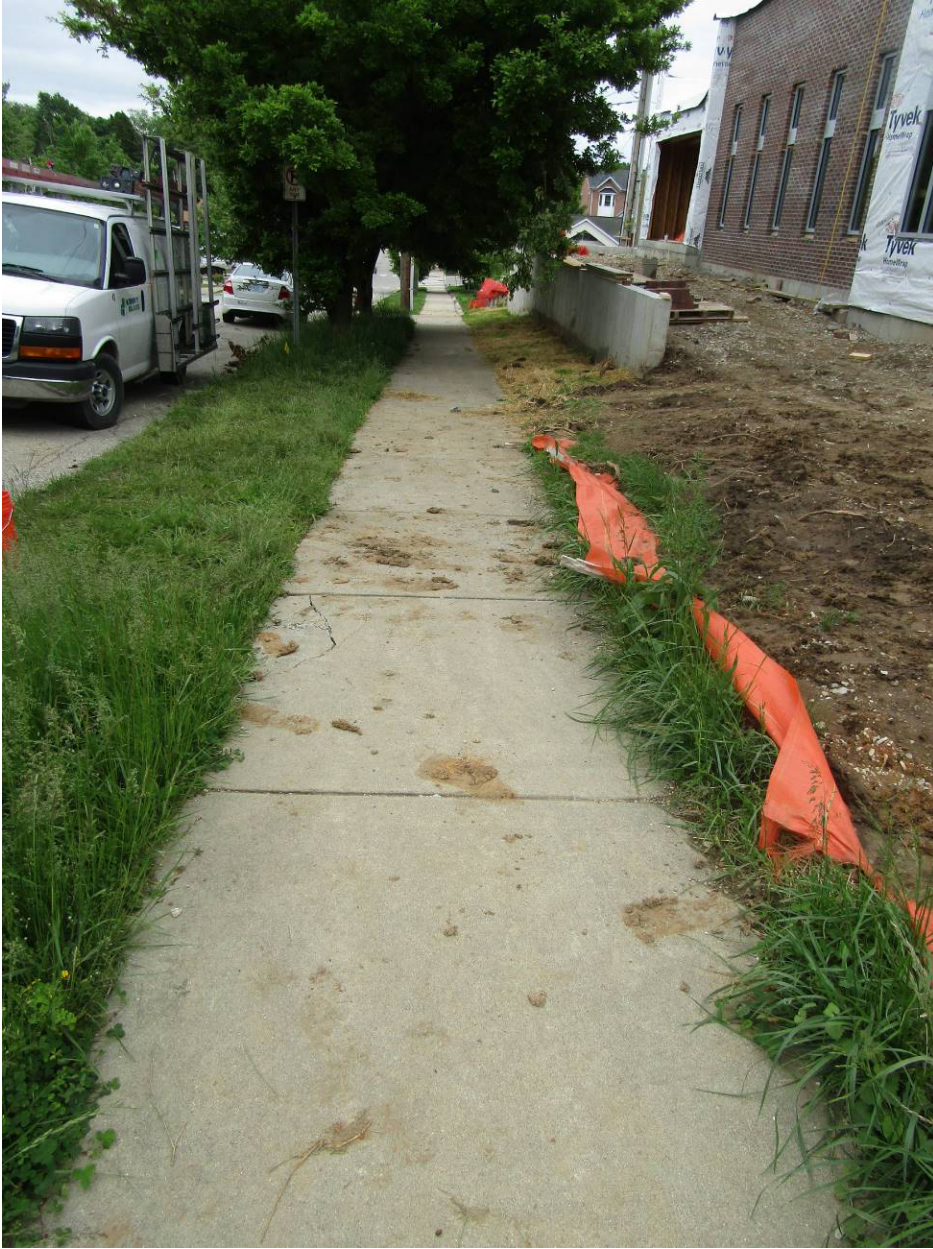
Figure 5: Silt fence failed; tracking onto the sidewalk.
