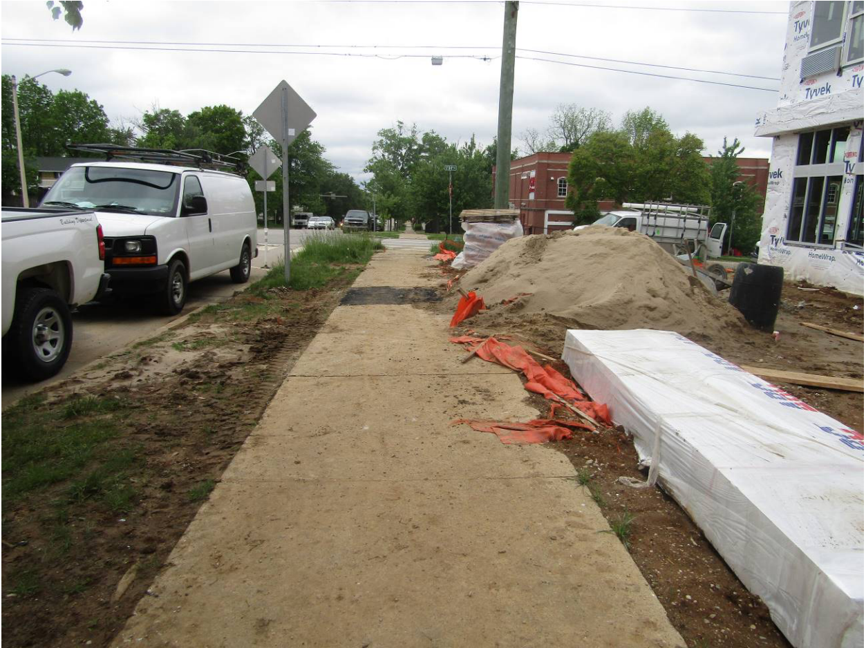
Figure 3: Silt fence collapsed and sediment tracked onto sidewalk.
