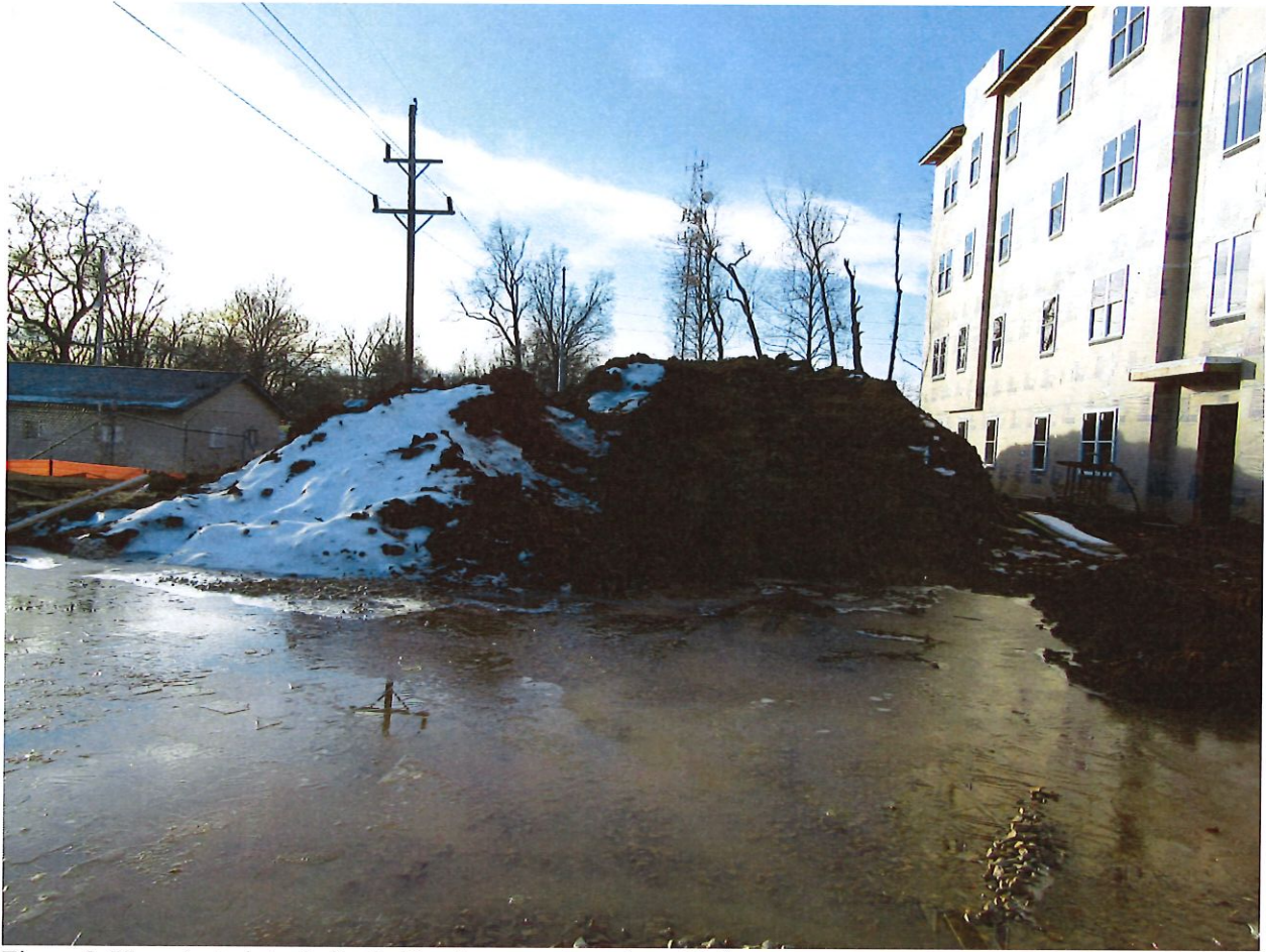
Figure 8: Unprotected stockpile that has been on site at least 10 days.
