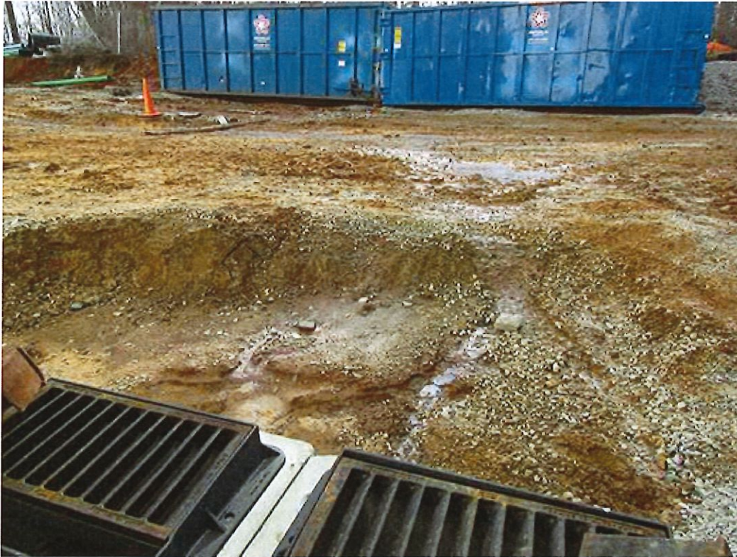
Figure 15: Unknown opaque white liquid seeping from dumpster area directly into the storm drains.
