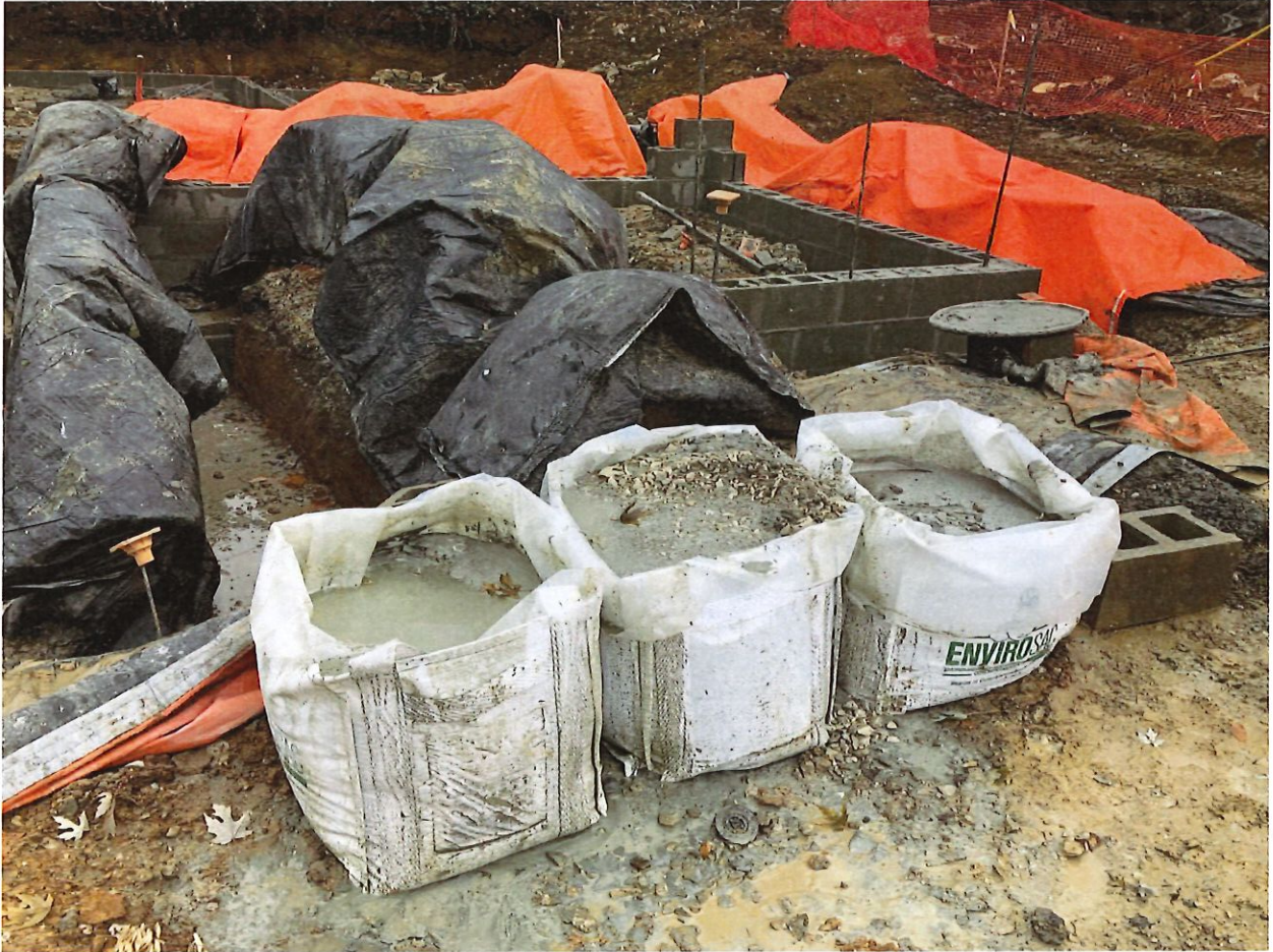
Figure 4: Improperly disposed of construction materials.
