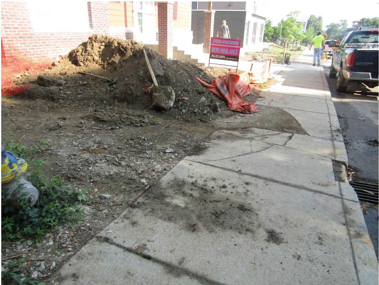
Figure 3: 7/6/2020 - Stockpile not properly protected along Walnut Street. Sediment on the sidewalk. This area of the project has been exposed for longer than 14 days.
