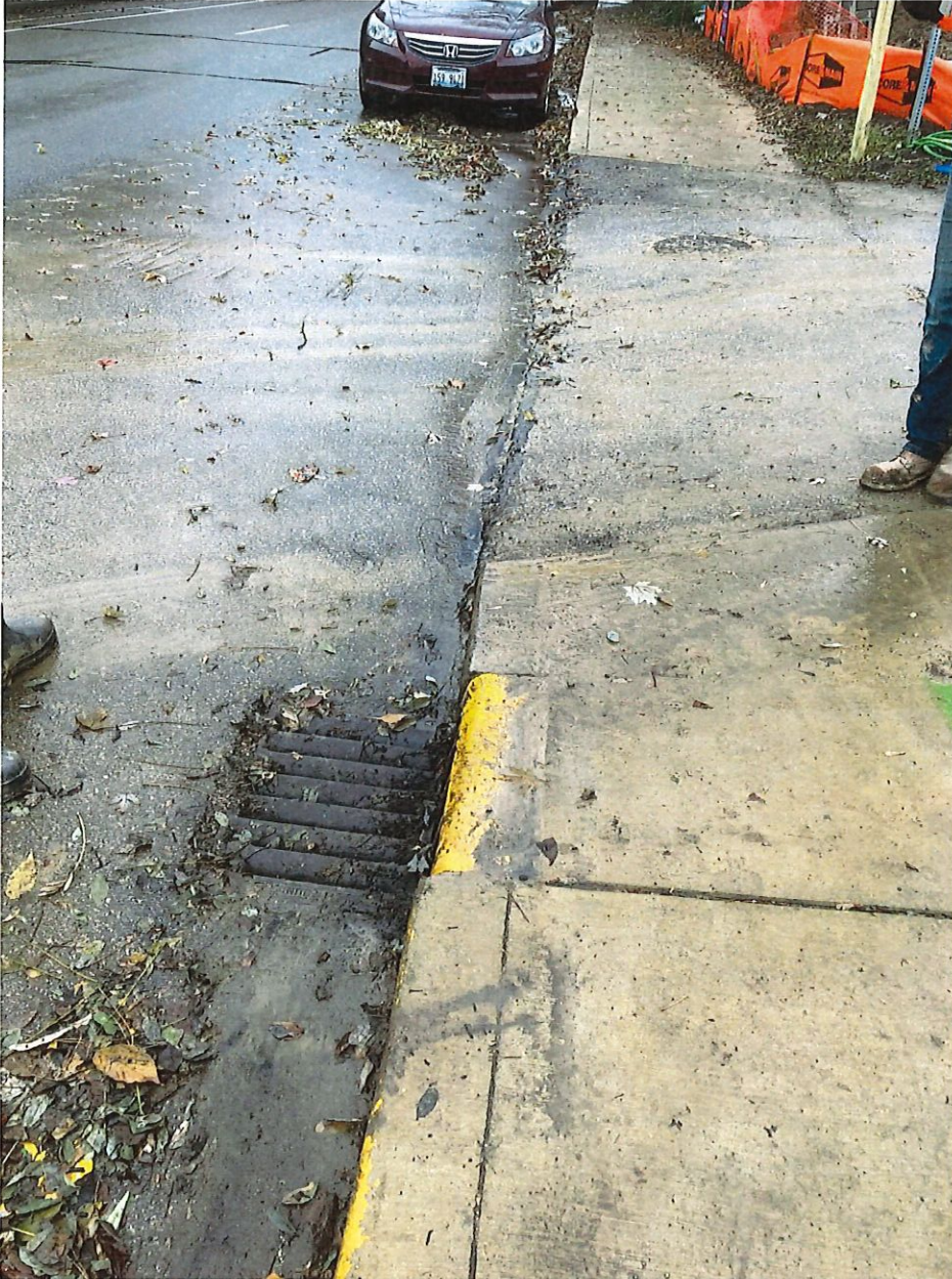
Figure 3: Tracking and unprotected storm drain inlet.
