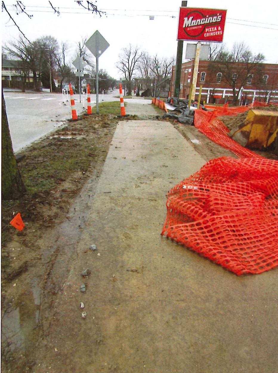
Figure 2: Mud tracked onto the sidewalk and into the street.
