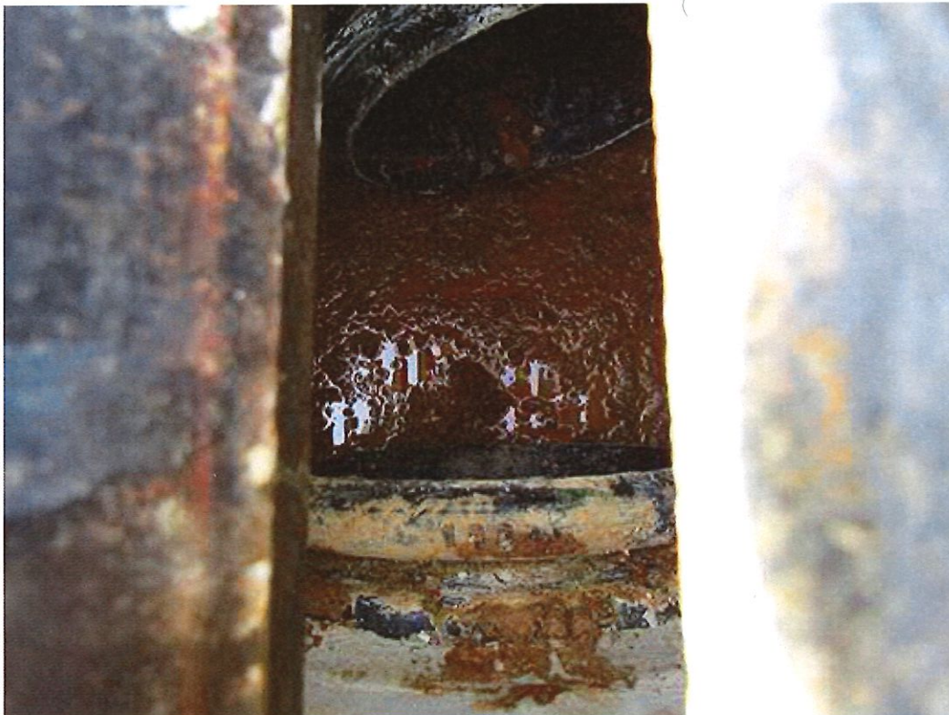
Figure 20: Sediment inside a storm inlet.
