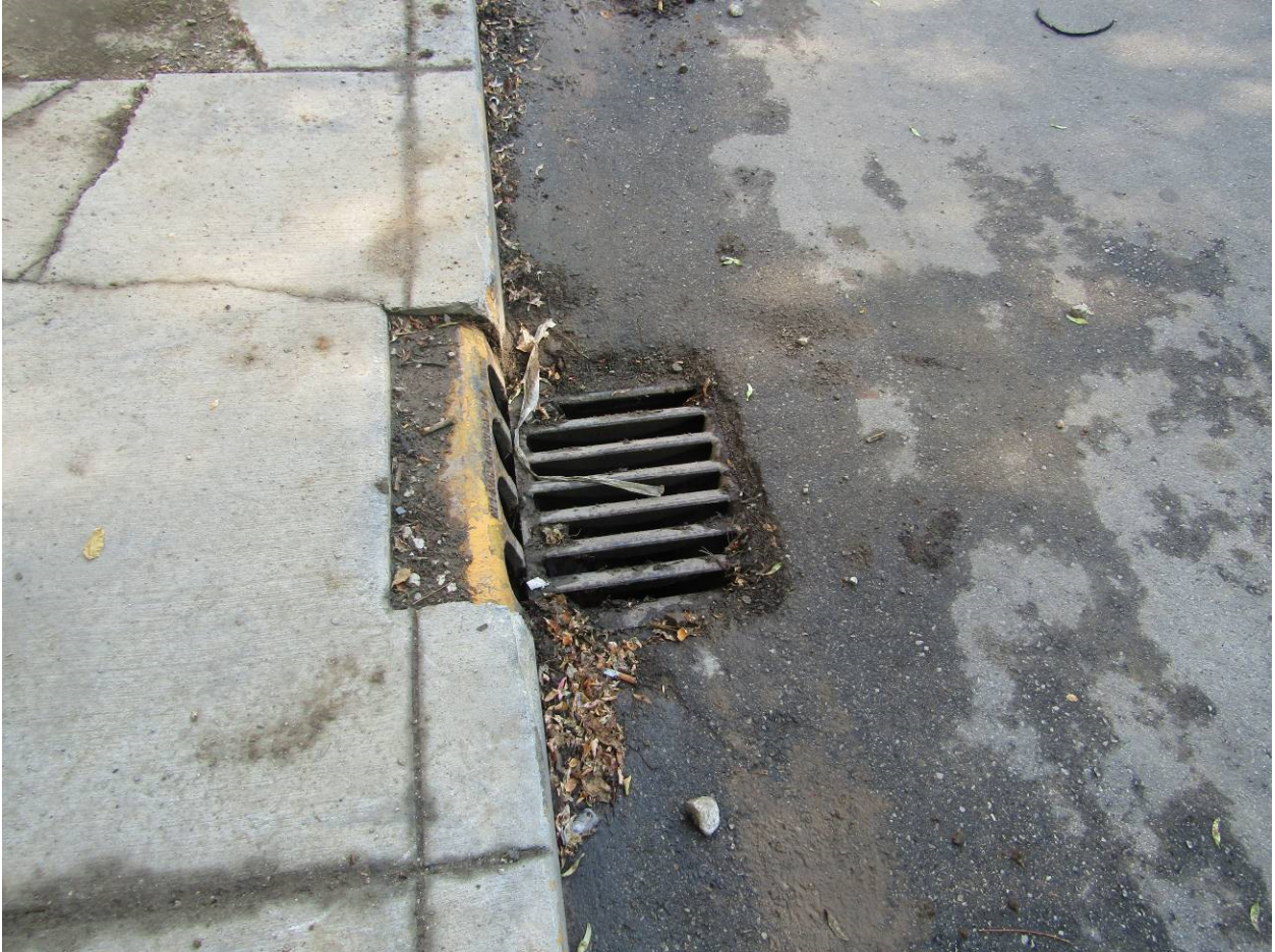
Figure 2: 7/6/2020 - Inlet south of the alley along Walnut Street not protected and with sediment immediately adjacent.
