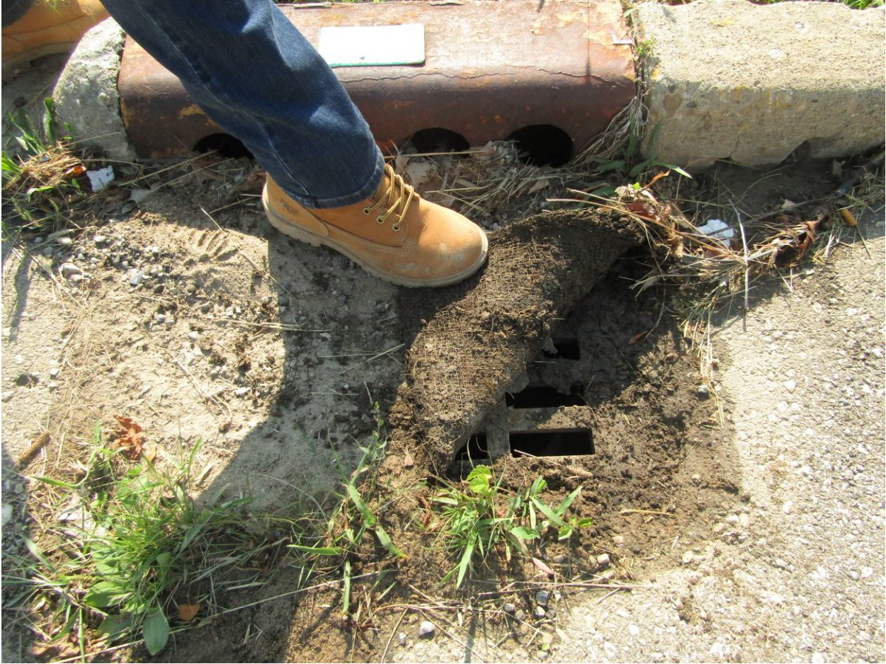
Figure 8: 7/6/2020 - Inlet along College Avenue has not been maintained/properly protected.
