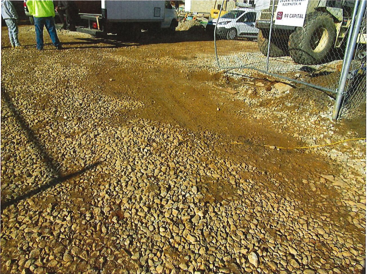
Figure 9: Muddy construction entrance.
