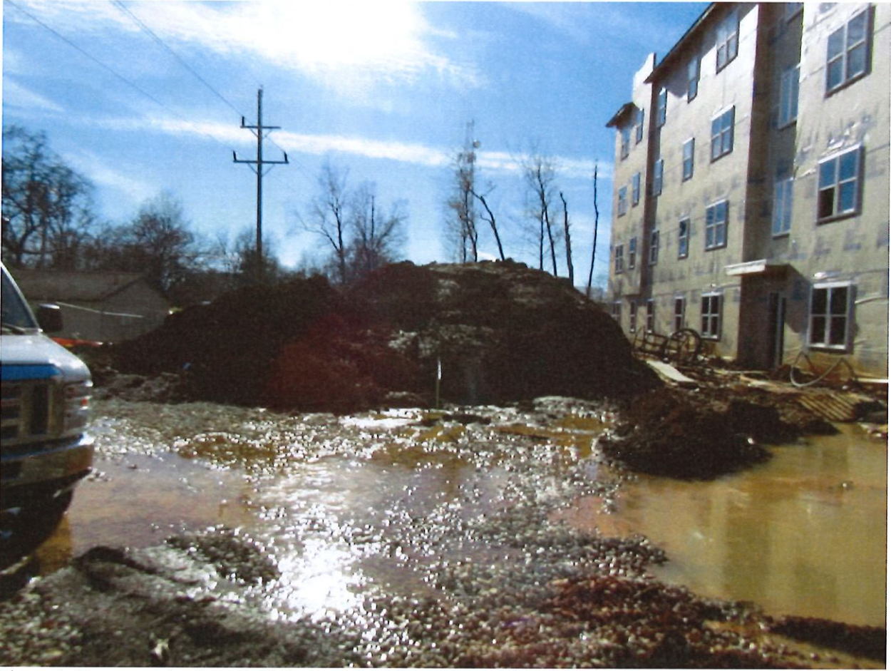
Figure 4: Unprotected soil stockpile has remained for over 3 weeks at least.
