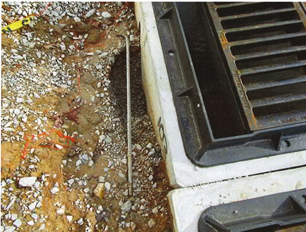
Figure 16: Sediment erosion around the storm inlet is causing sediment to flow directly into the inlet.
