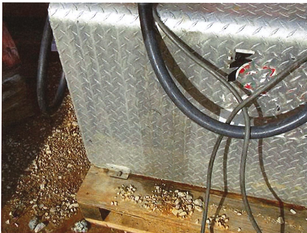
Figure 14: Leaking/spilled fuel running down the sides of the fuel tank and collecting on the pallet.
