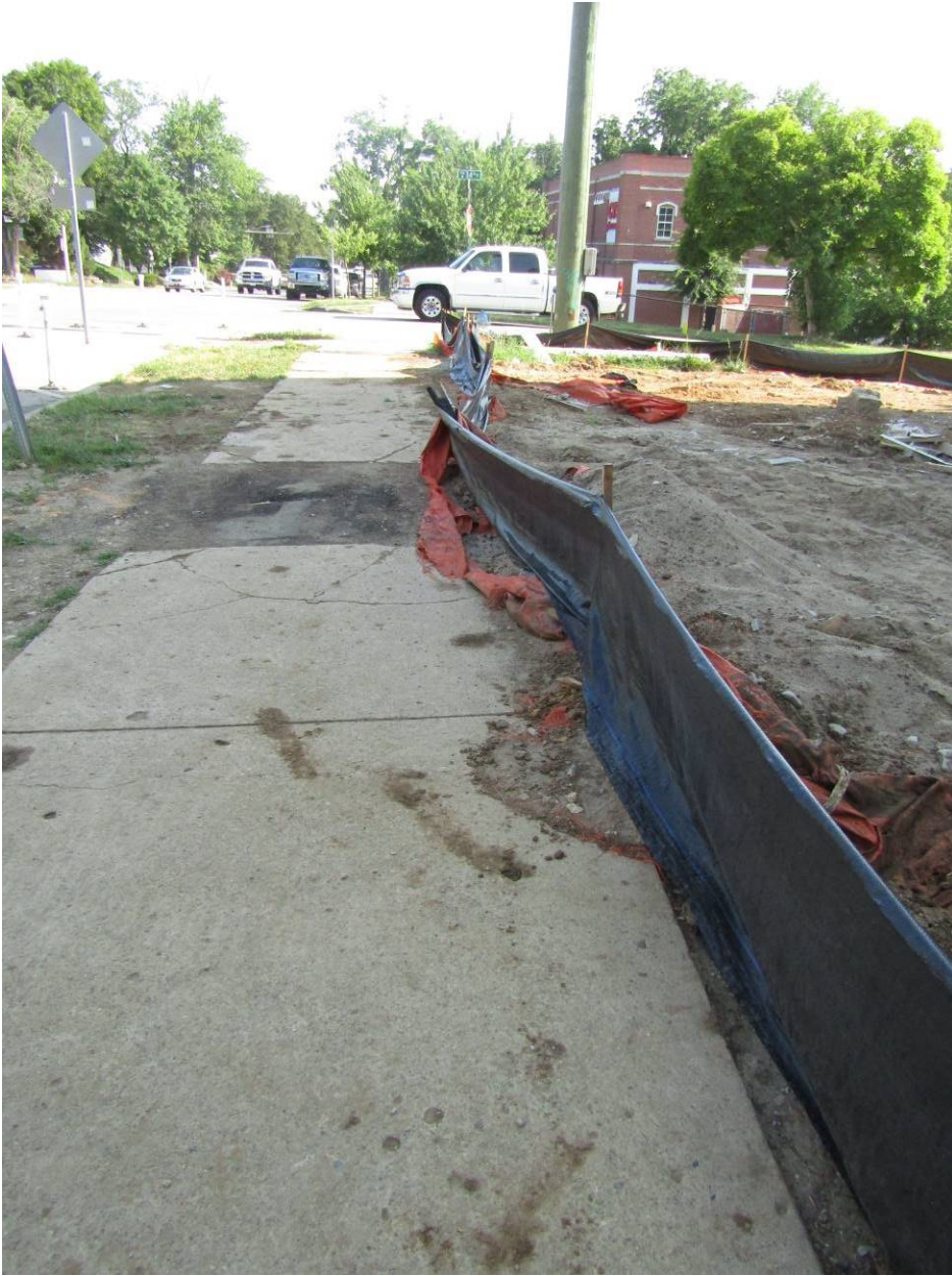
Figure 7: 7/6/2020 - Silt fence not installed properly along College Avenue. Sediment is not being contained to the site and has been tracked into the sidewalk.
