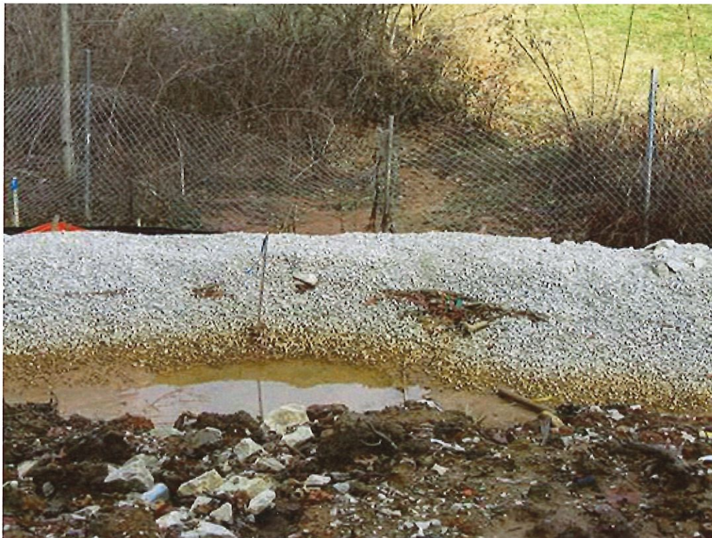
Figure 22: The upper basin of the structure is full of sediment and not working effectively.
