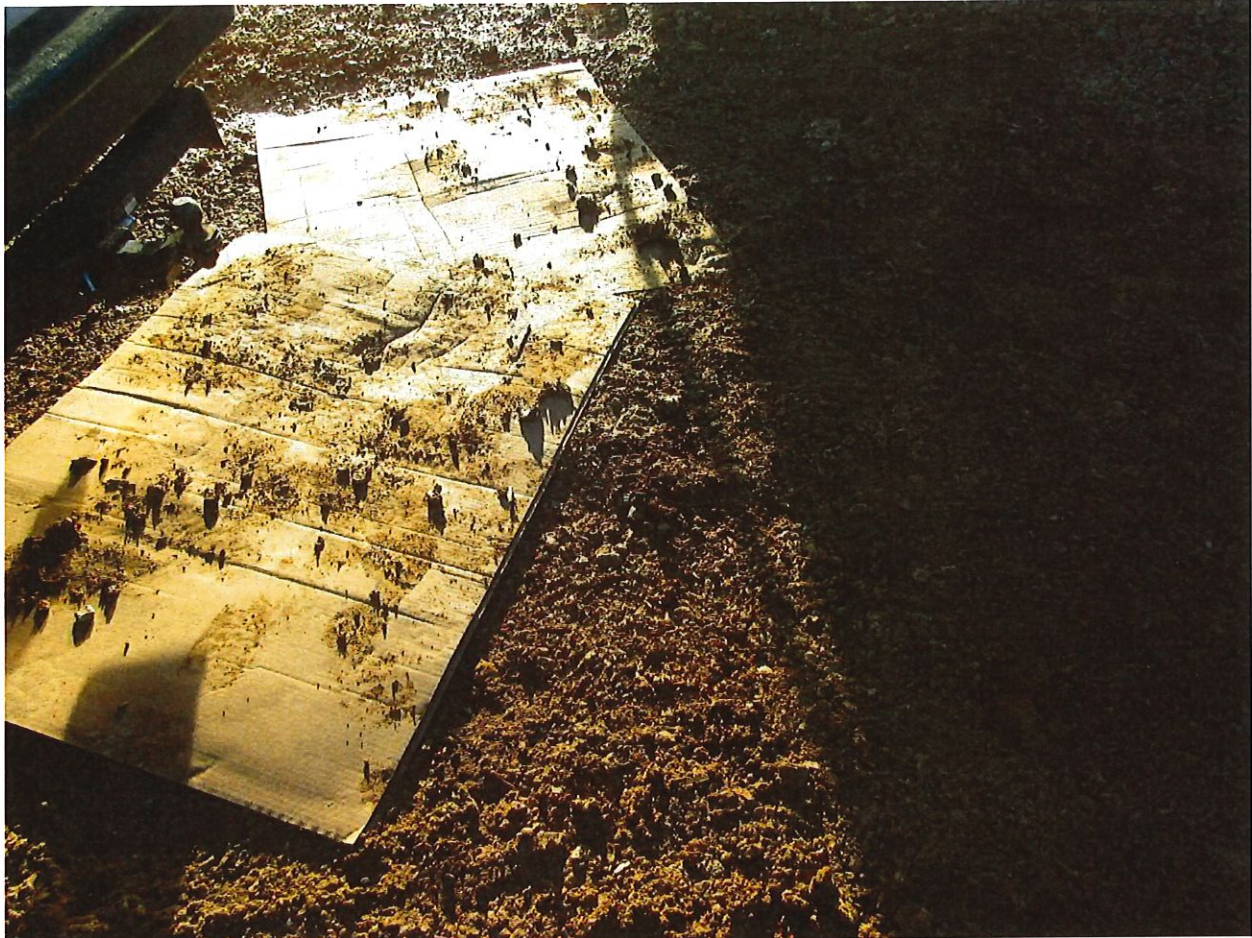
Figure 5: Muddy parking area. Subcontractors are improvising so that they do not unload tools/equipment into the mud.
