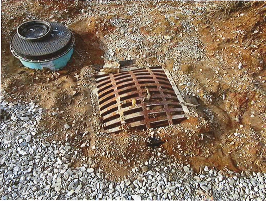
Figure 17: Filter fabric is in place, but needs maintenance.
