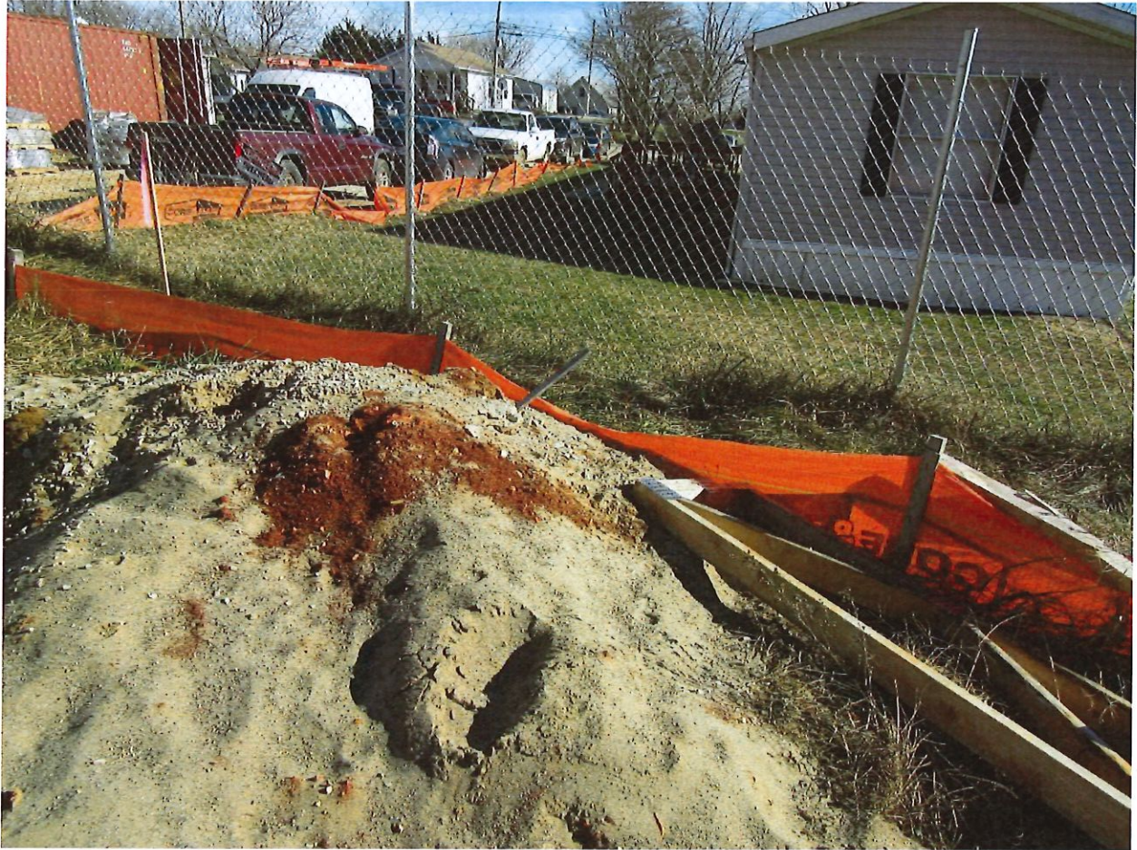
Figure 6: Improperly disposed of/contained materials immediately adjacent to a failing silt fence.
