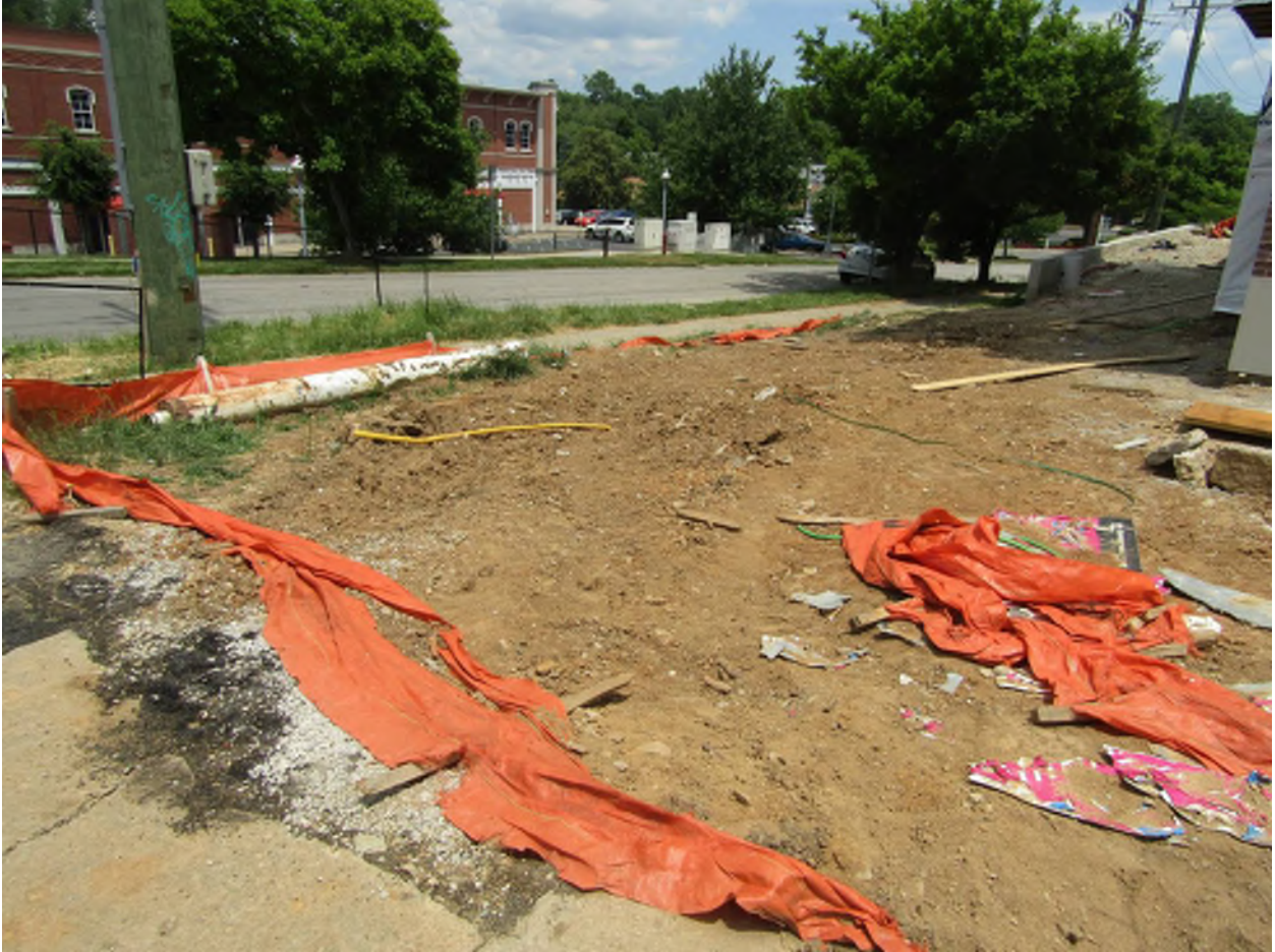
Figure 4: Silt fence collapsed; tracking onto the sidewalk.
