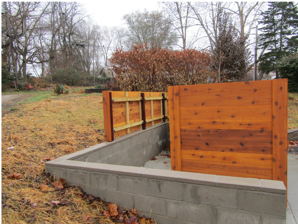
Figure 1: Dumpster is not enclosed on all sides with a minimum 6 foot enclosure.
