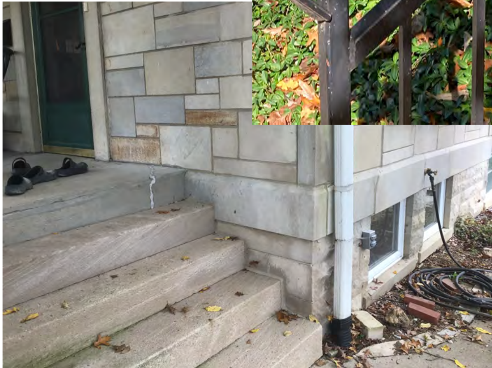
1014 E. Wylie Street - Front Steps
