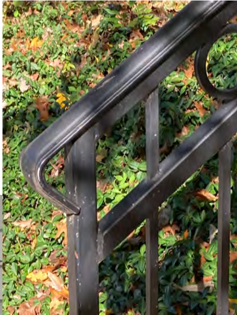
1014 E. Wylie Street - Existing Lower Guardrail
