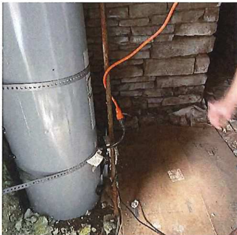
Women's House: Extension cord in Italianate basement.
