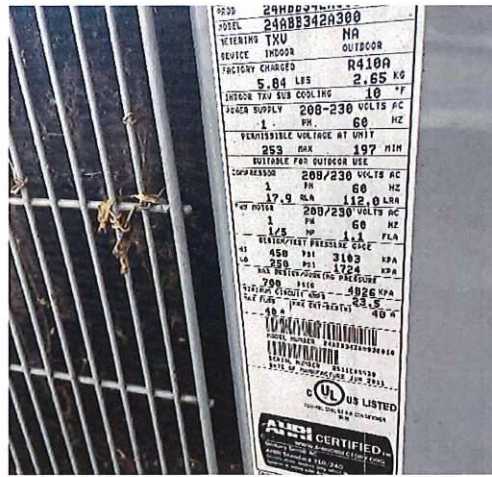
Women's House: Inefficient mechanical equipment.
