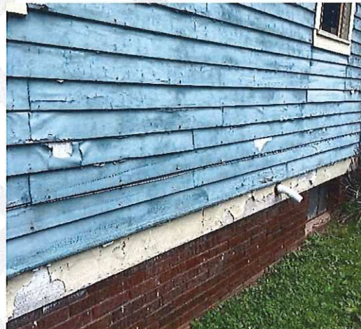
Women's House: deteriorated paint at Bungalow.
