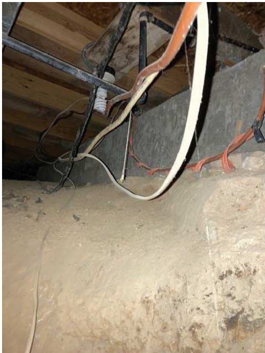
Old foundation repair under I-wing (completed by unknown previous owner)
