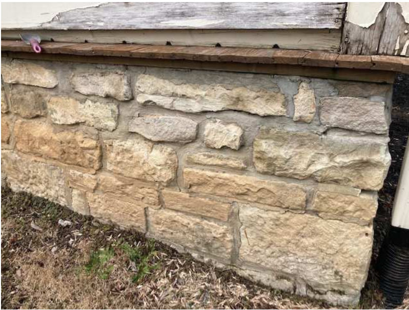
Stone pointing shows evidence of multiple repairs and cracking
