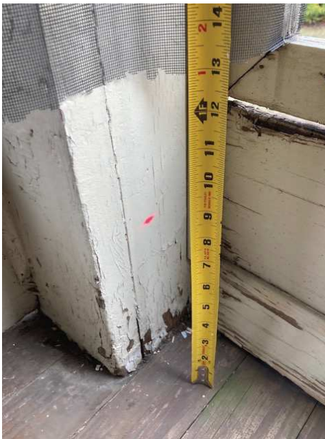
9" of vertical drop in 21' (measured from opposite corner)
