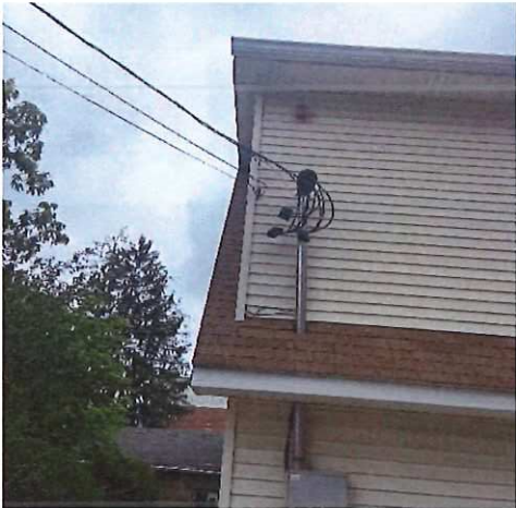
Men's House: No flashing at roof penetration.
