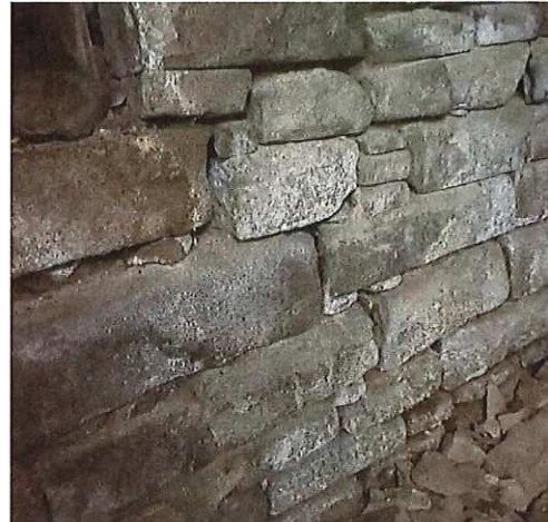
Women's House: Deterioration of mortar in Italianate basement walls.
