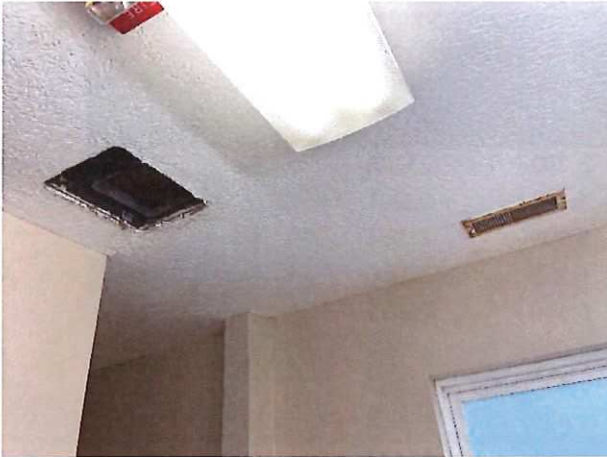
Men's House: Second floor bathroom, lack of exhaust fan with rusted vent visible.
