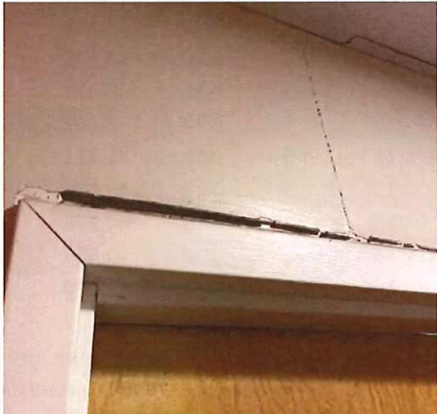
Men's House: "Dropped" door frames and "popped" drywall.
