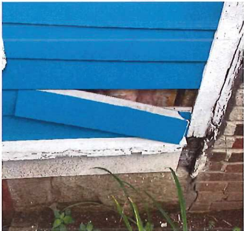
Men's House: Lack of sheathing under clapboards (Board was already loose when we did the site visit).
