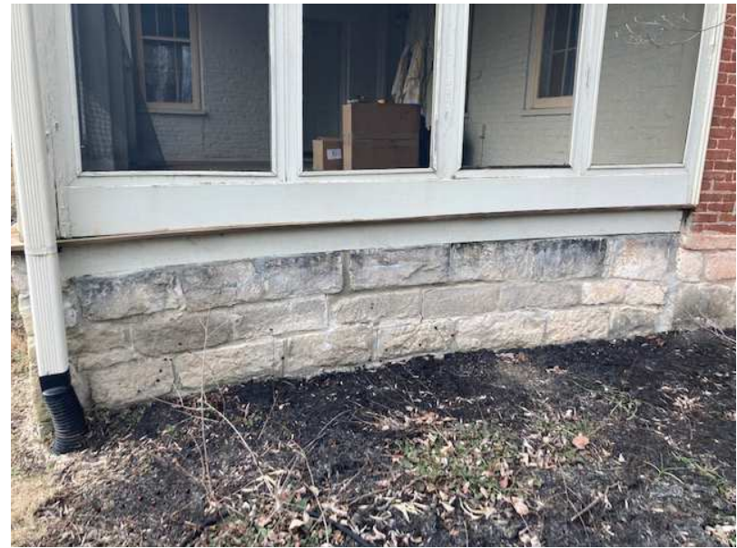
Side view showing bending of foundation stones and beam supporting porch.
