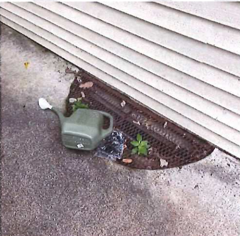
Men's House: Concrete slab is above vinyl cladding.
