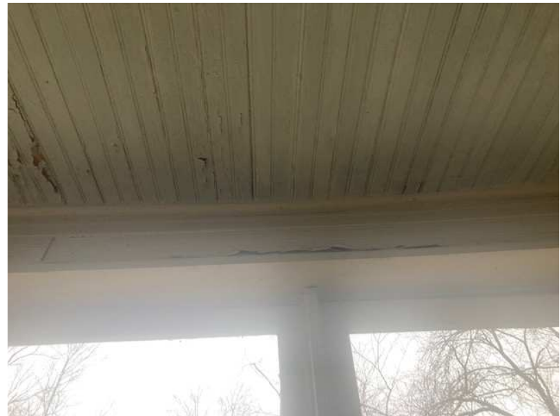
Interior view of bent support beam. Multiple contractors advised that replacement not feasible
