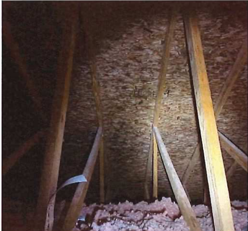
Men's House attic: Possible mold forming on north roof sheathing.
