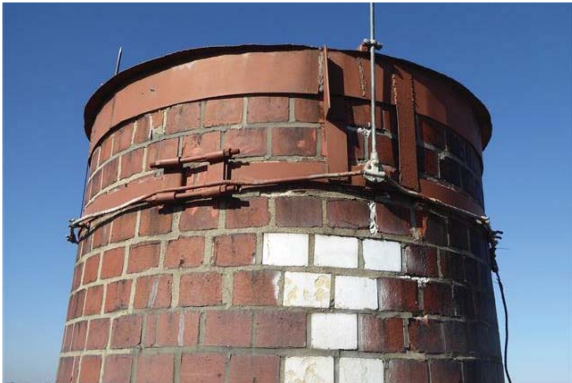
Photo 12 This prevents rain from falling inside but promotes freeze/thaw deterioration due to the “chimney effect” where warm, moist air rises and condenses on the inside face of the masonry.
