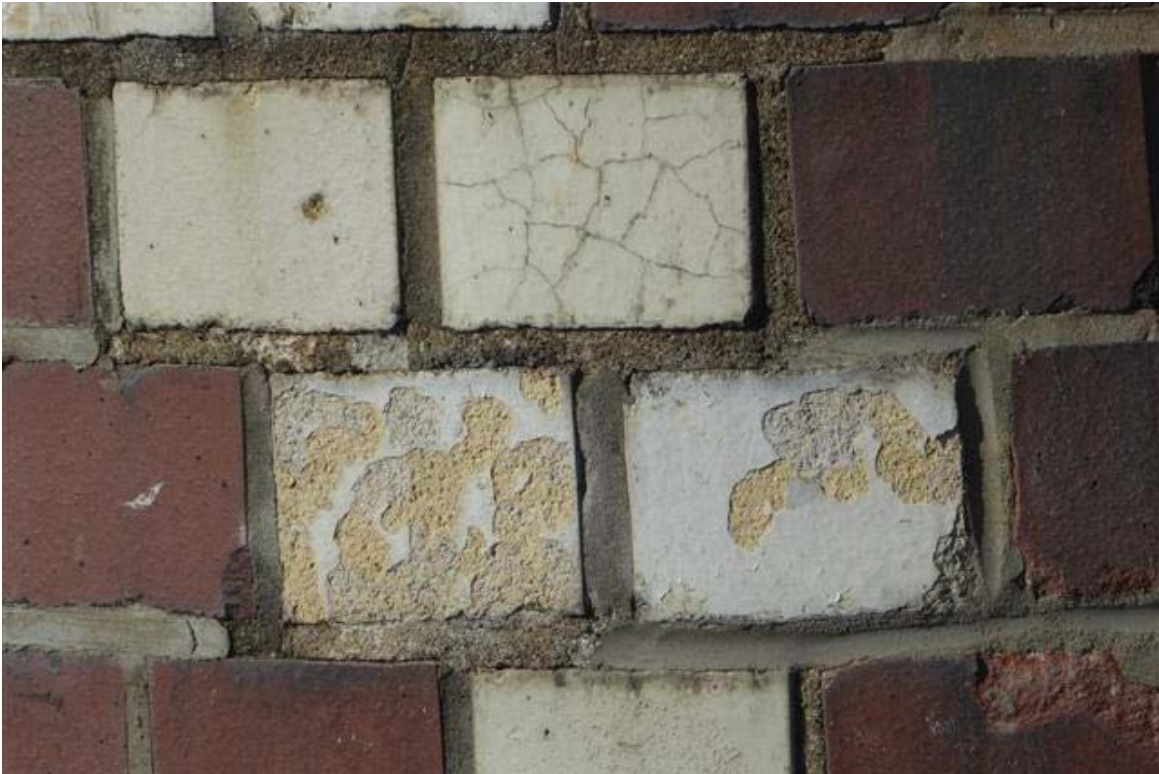
Photo 29 Glaze spalls continue to occur.
