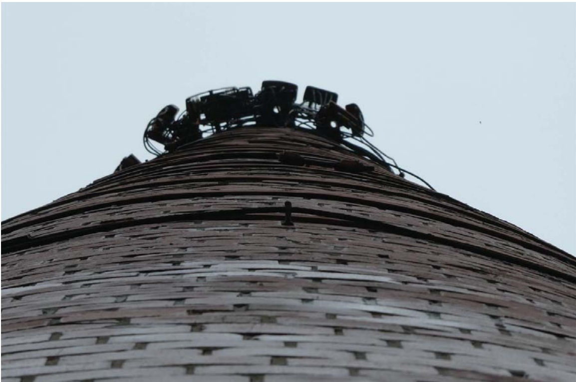
Photo 2 Looking up the wall of the stack on the opposite side as Photo 1.
