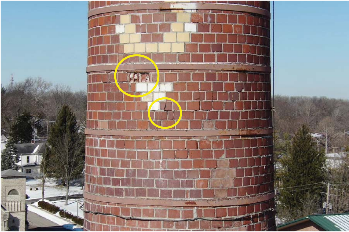
Photo 5 New spalls are highlighted in this 2022 photo.
