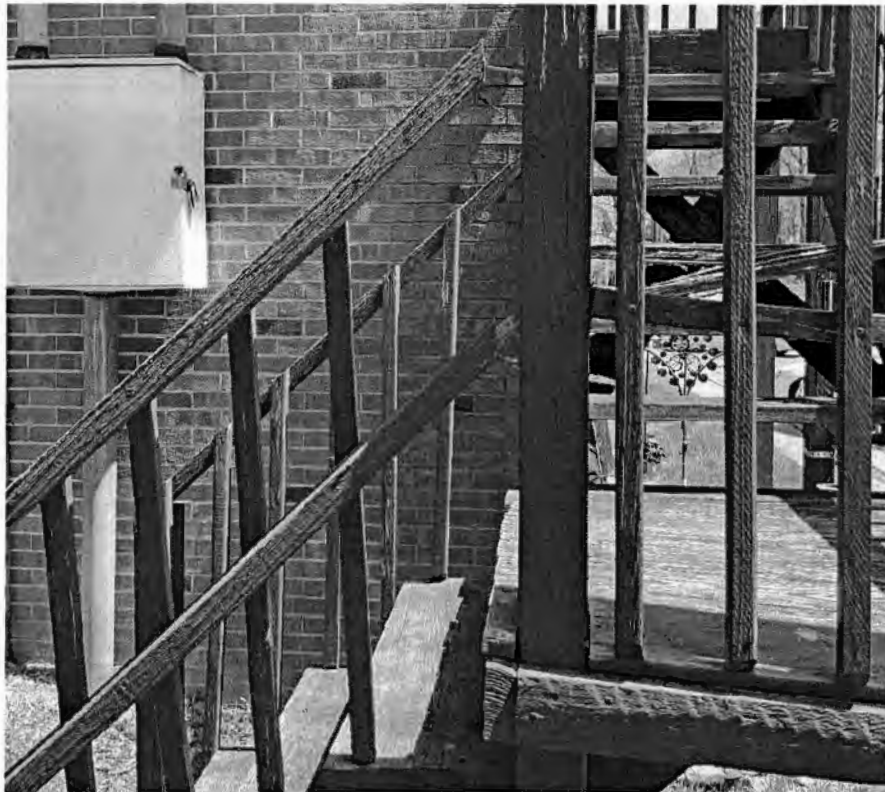
Example of loose handrail and missing spindles
