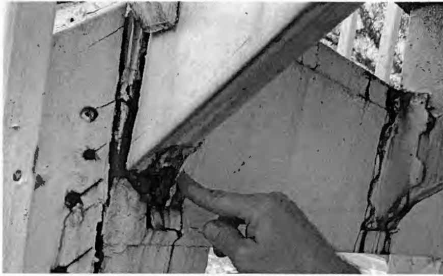
Example of deteriorated joist hanger
