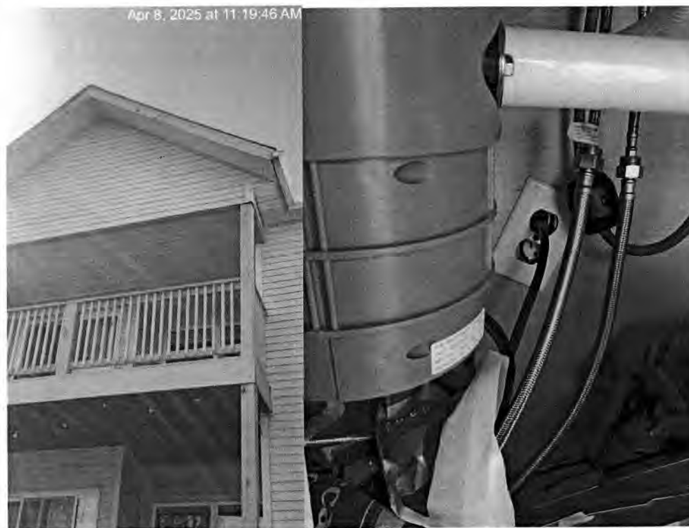
Building 2931: Top left - loose junction box, no conduit. Top right - Some of the damage siding. There was also missing siding (no picture). Bottom left - Missing metal fascia. Bottom Right - example of set back outlets under sink cabinets.
