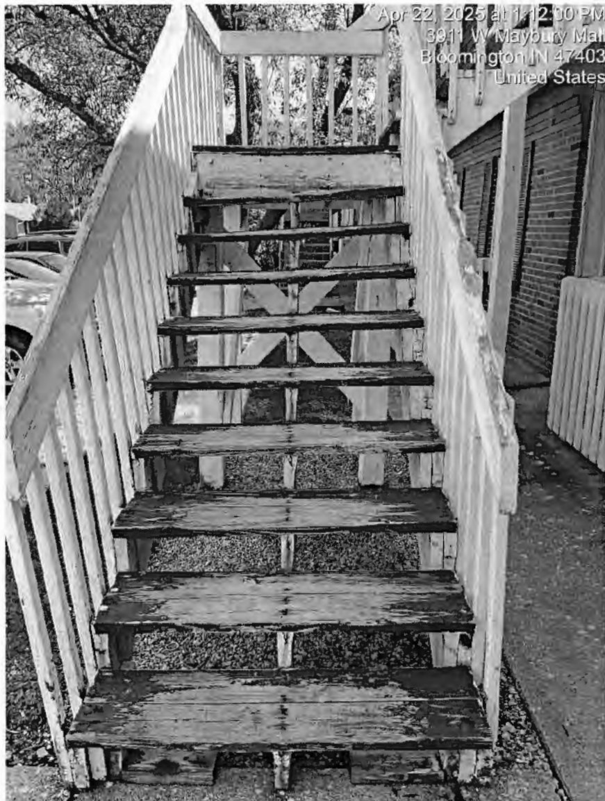
Example of leaning/listing stair
