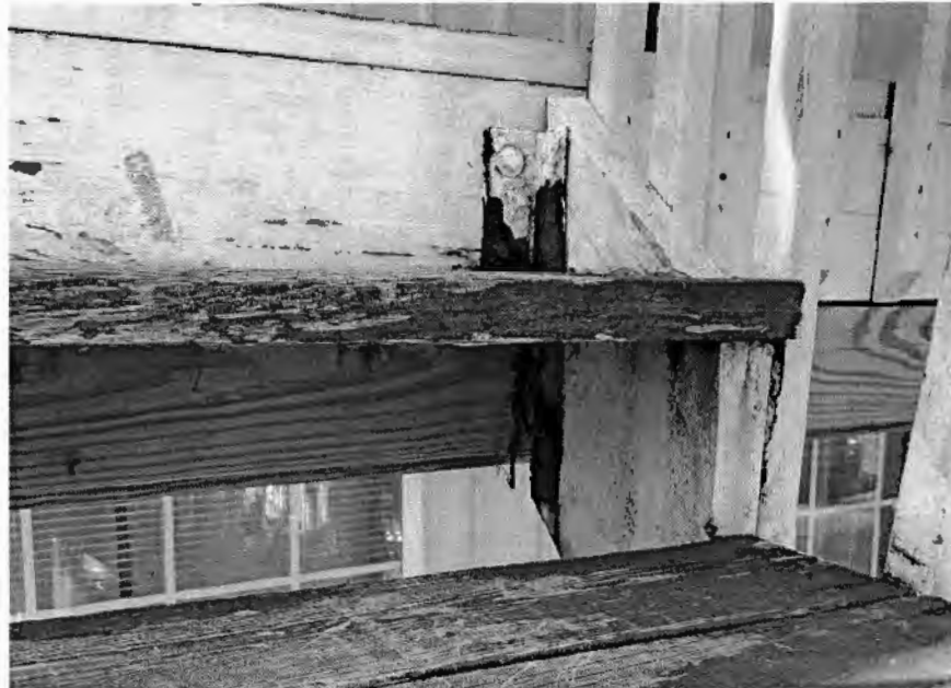
Example of deteriorated brack
