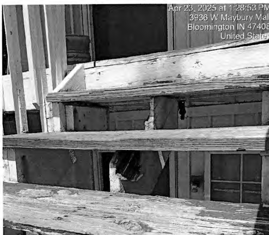
Example of deteriorated stringer
