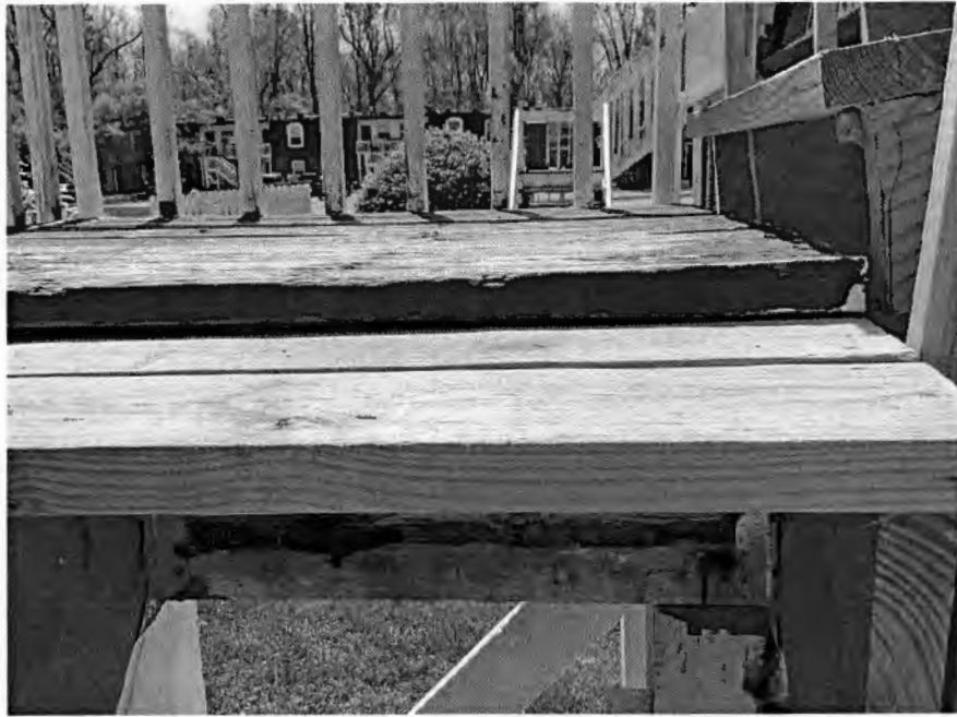
Example of trip hazard
