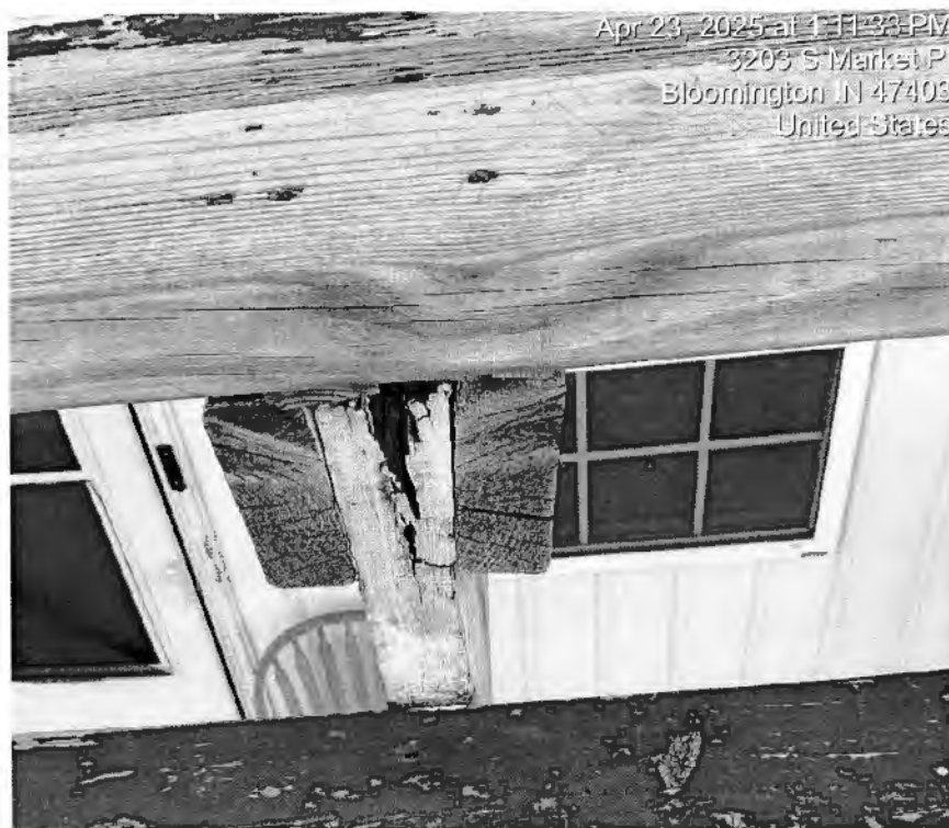
Example of deteriorated stringer
