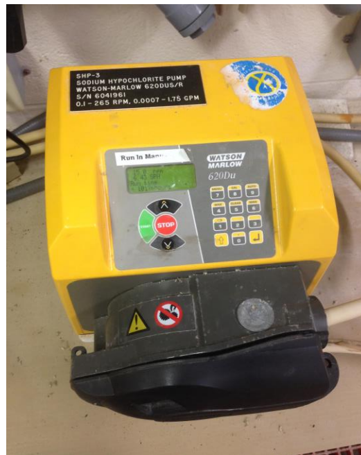
At the Dillman Road WWTP, sodium hypochlorite is used to disinfect water. Ultra-violet (UV) light is used to disinfect water at Blucher Poole WWTP.
