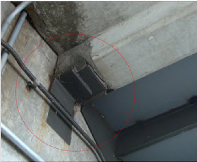
REPAIR ID - 02B
