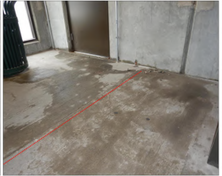
REPAIR ID - 15C
