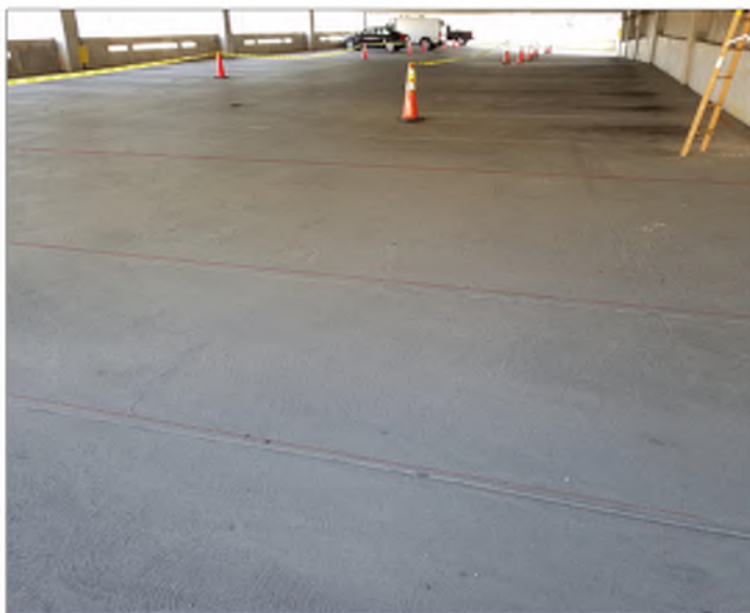
REPAIR ID - 9C
