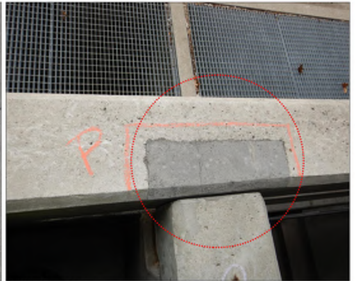
REPAIR ID - 10F
