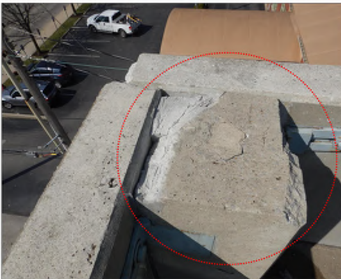
REPAIR ID - 10D
