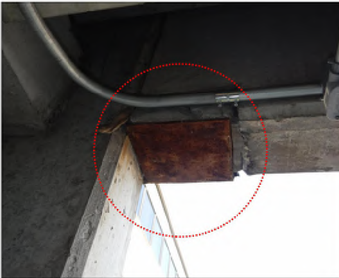
REPAIR ID - 11D
