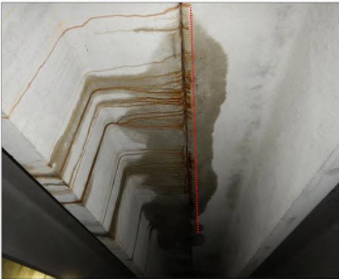
REPAIR ID - 12B
