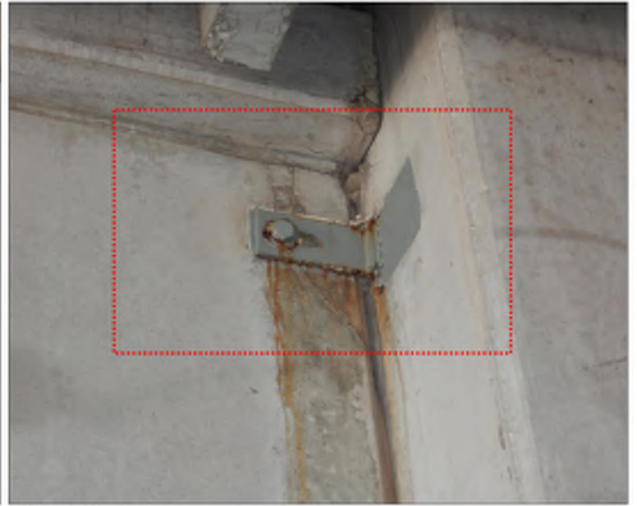
REPAIR ID - 05D
