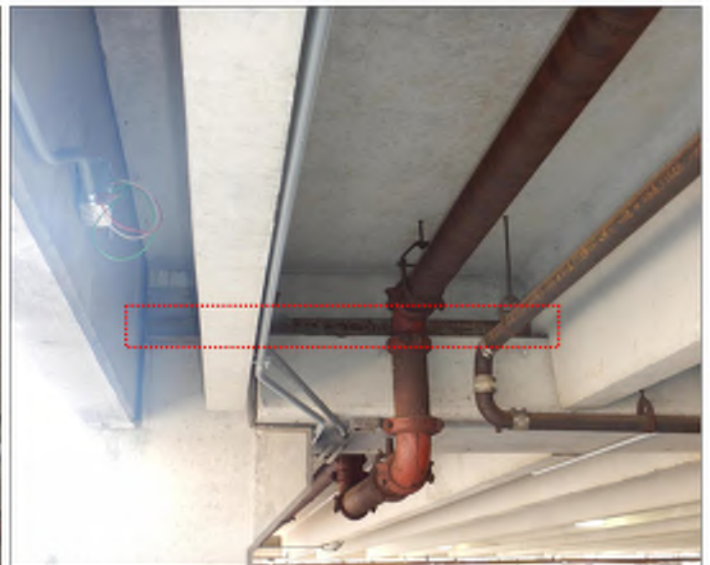
REPAIR ID - 05B
