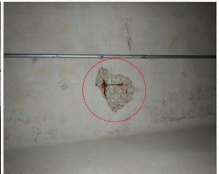
REPAIR ID - 03C
