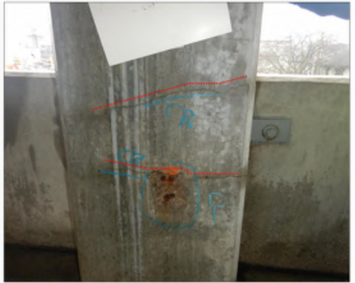
REPAIR ID - 07C
