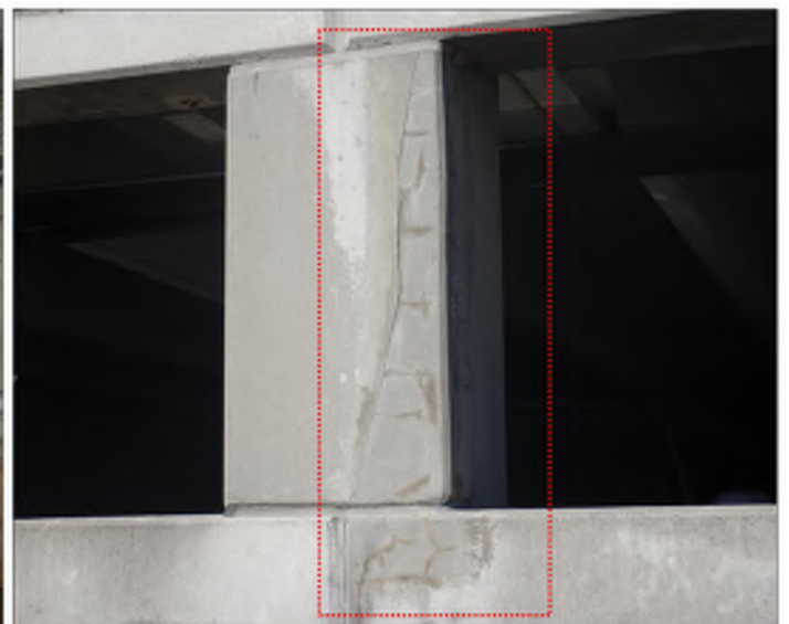
REPAIR ID - 11C
