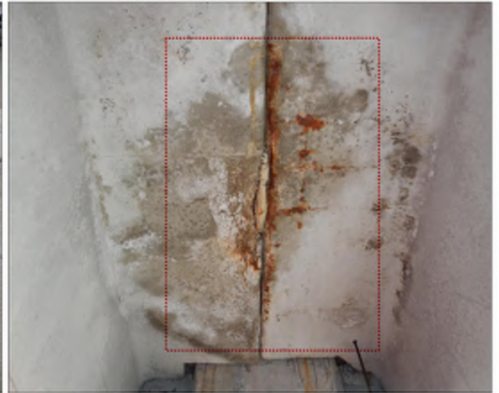
REPAIR ID - 10C
