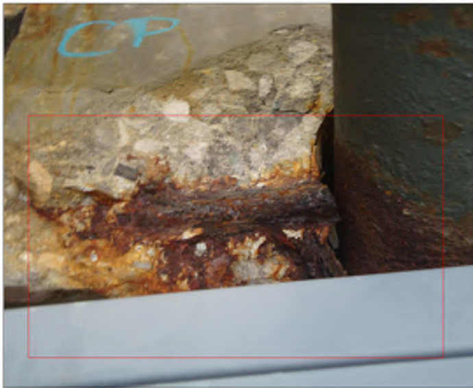
REPAIR ID - 03F
