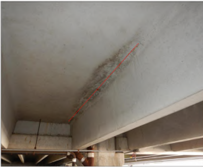
REPAIR ID - 07B-2
