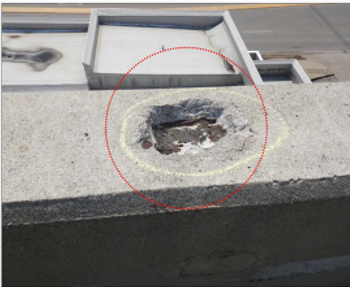
REPAIR ID - 03B
