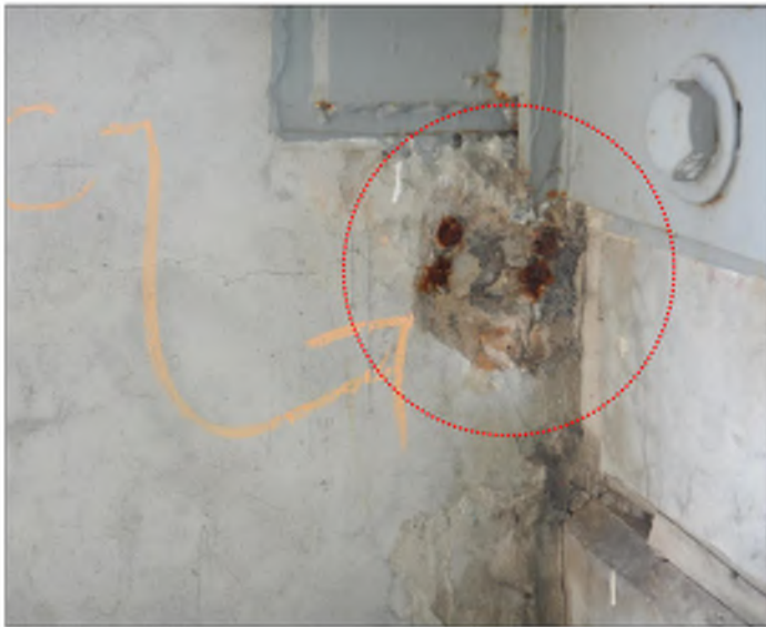
REPAIR ID - 03D
