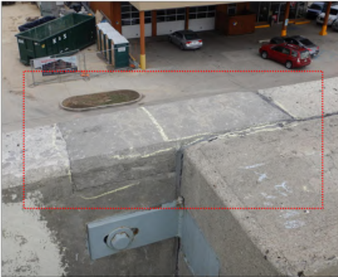
REPAIR ID - 10B
