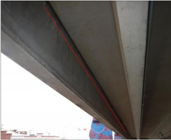
REPAIR ID - 09B
