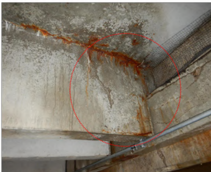
REPAIR ID - 11B
