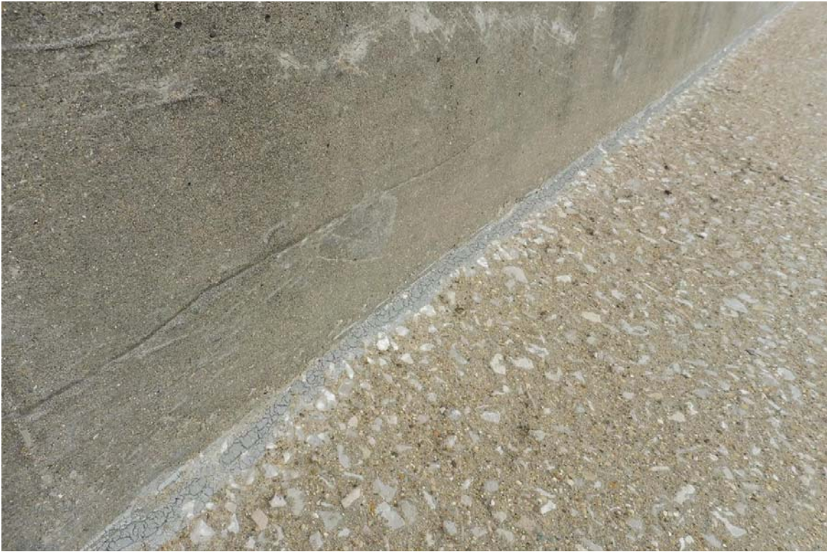
Photo 71 The perimeter sealant joints, however, are in fair to poor condition as many have failed such as the joint seen here on the roof level.
