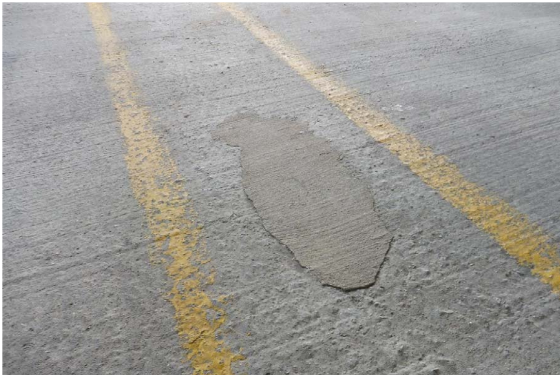
Photo 74 The floor slabs are in good condition while few existing patches were observed. The existing patch seen here was unsound and should be repaired.
