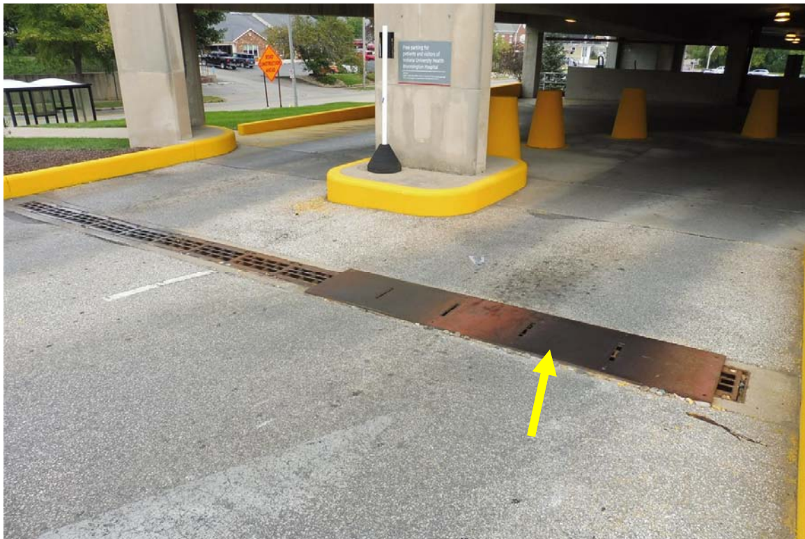
Photo 78 Steel road plate installed over the trench drain at the main entrance. The plate was loose and needs to be re-anchored. The condition of the trench drain below the road plate was not visible.
