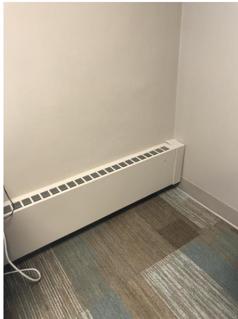
Perimeter hot water heater
