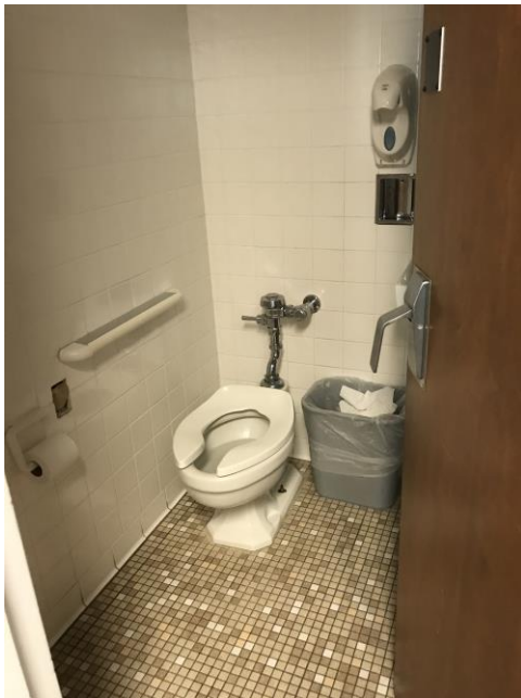
Typical water closet
