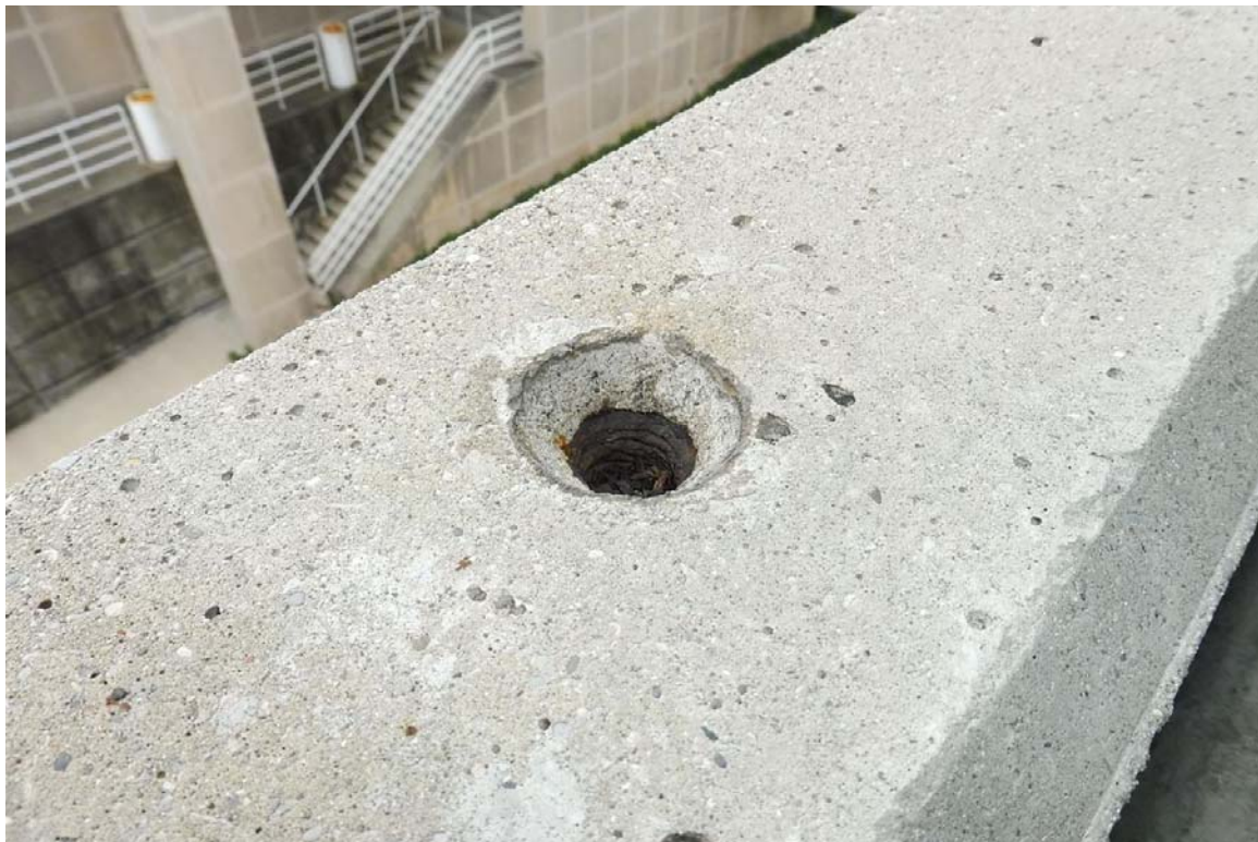
Photo 88 ...should be cleaned and filled with non-shrink grout to keep the metal insert embedment from corroding.
