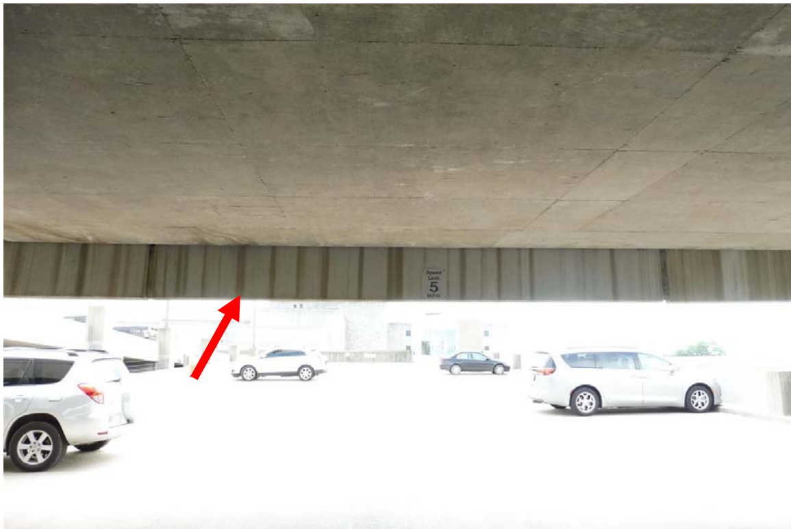
Photo 72 Staining on the back face of the edge spandrel is the result of water migration through the failed perimeter sealant joint above on the roof level.
