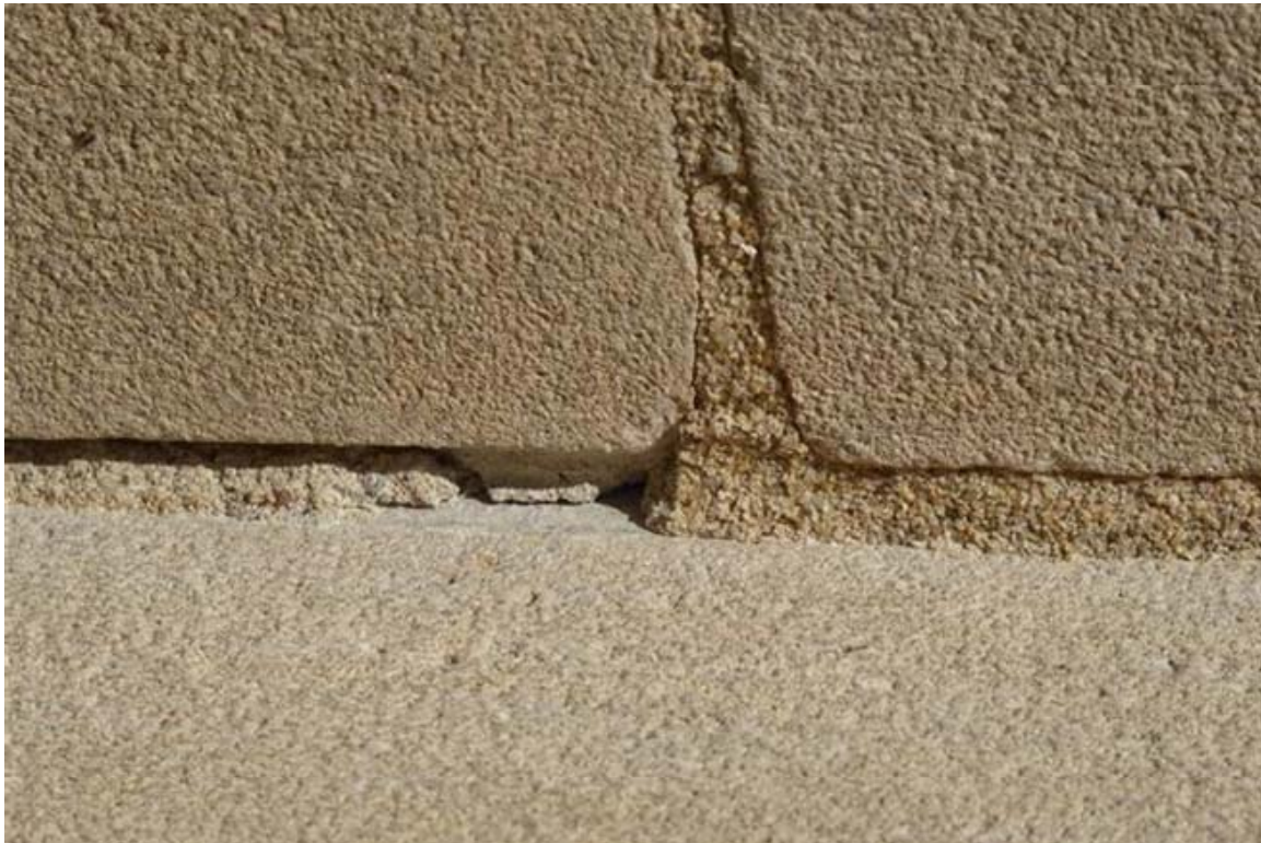
Photo 26 More recent tuckpointing has been thin and tends to crack and fall back out of the joint.
