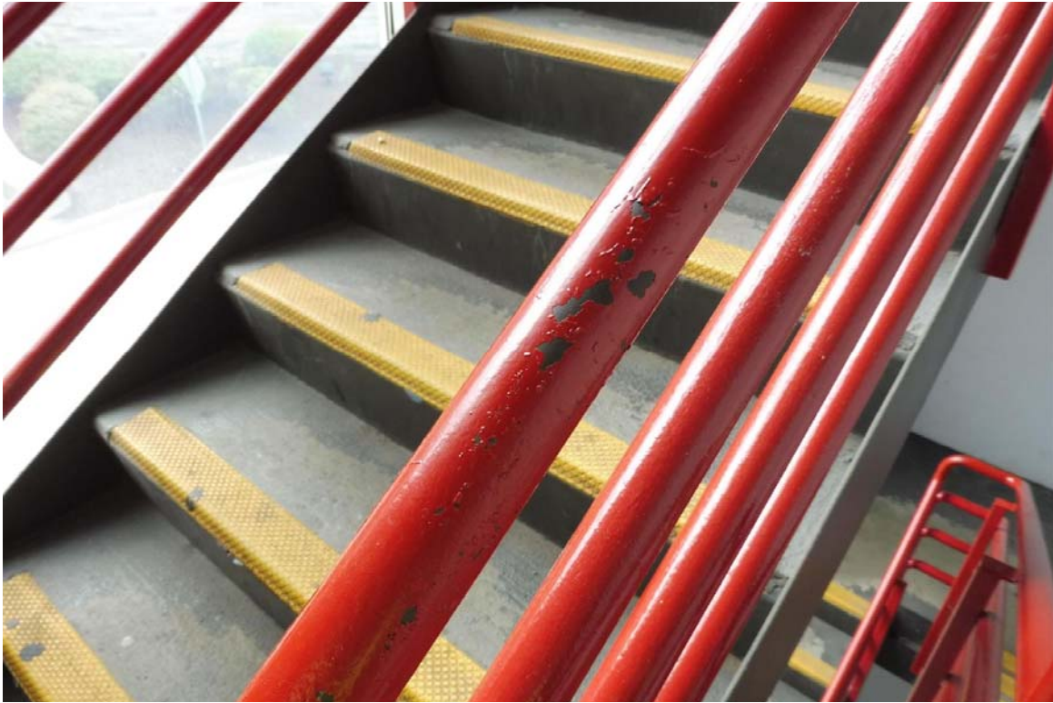
Photo 109 The paint system on the handrails was generally in good condition with few areas as seen here where the coating is starting to fail.
