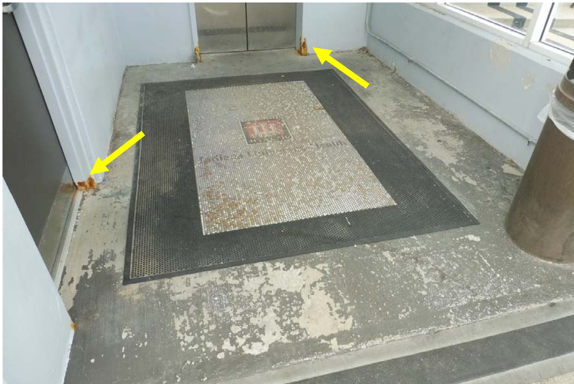
Photo 100 The existing floor coating throughout the stair/elevator tower has failed. Corrosion of the door frames both to the stair and the elevator were observed on each level.
