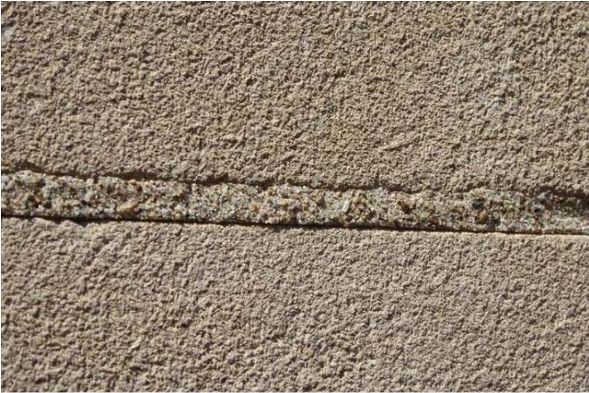
Photo 25 A few of the joints were struck flush and are more prone to moisture infiltration.
