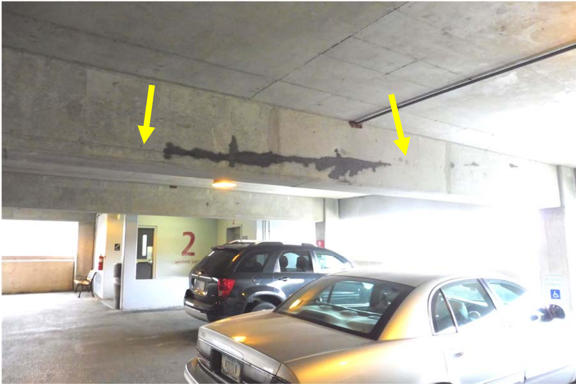
Photo 65 Level 3 beam seen from standing on Level 2 where grease from the tendons has leached out of the crack in the face of the beam.
