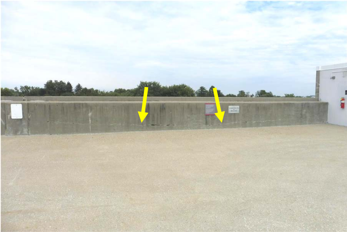
Photo 63 Post-tensioned beam along the north elevation at the roof deck has a crack that appears to follow the drape of the post-tensioning tendons. Grease is leaching from the crack near midspan, meaning that the sheathing has failed possibly due to moisture entering the unbonded tendons.
