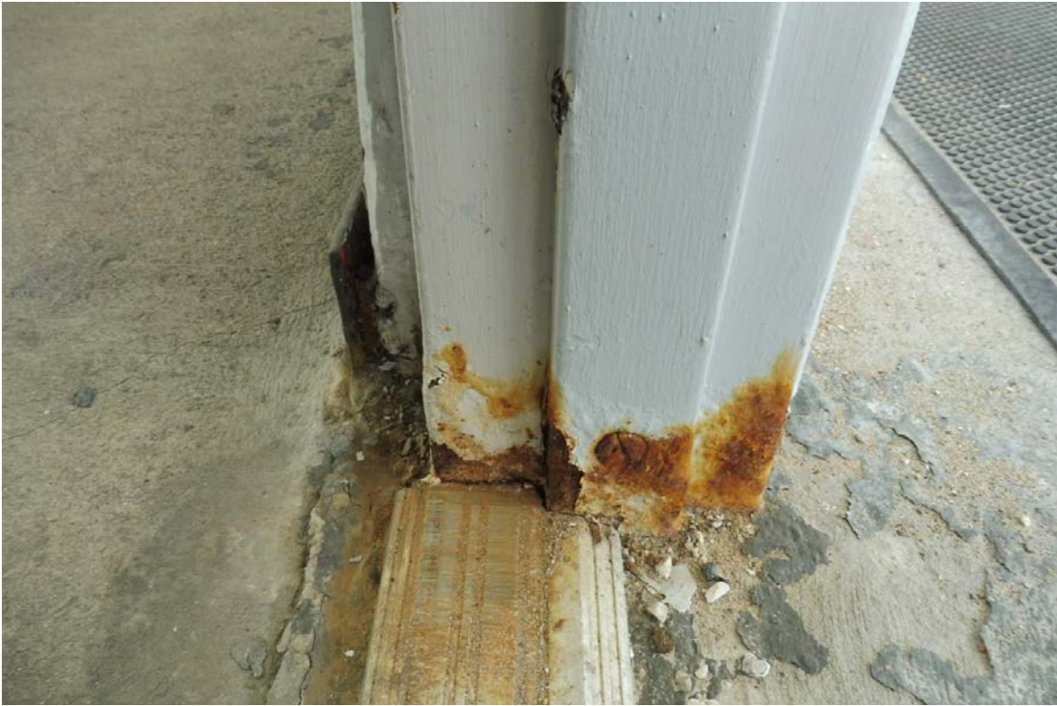
Photo 103 Corrosion at the bottom of the door frames...
