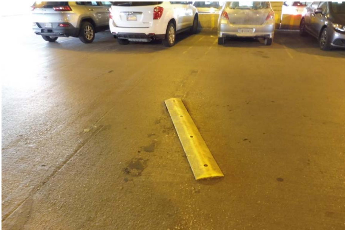
Photo 82 Speed bump devices have been installed. Several were missing and others were loose as seen here.
