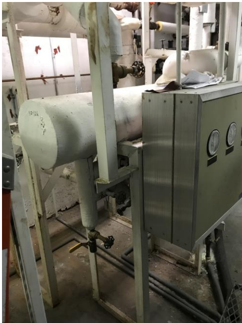
Steam-to-Hot Water Heat exchanger
