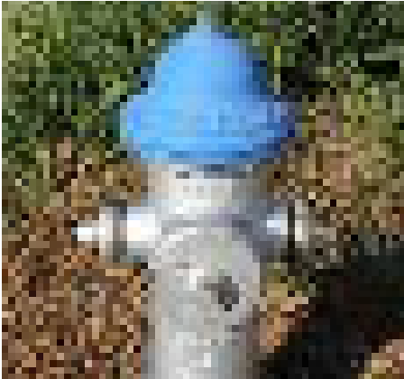
The approximately 2,944 fire hydrants owned and maintained by the Utilities Department provide the needed water flows for fire protection.
