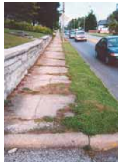
W. 2 nd St.: poor sidewalks and traffic
