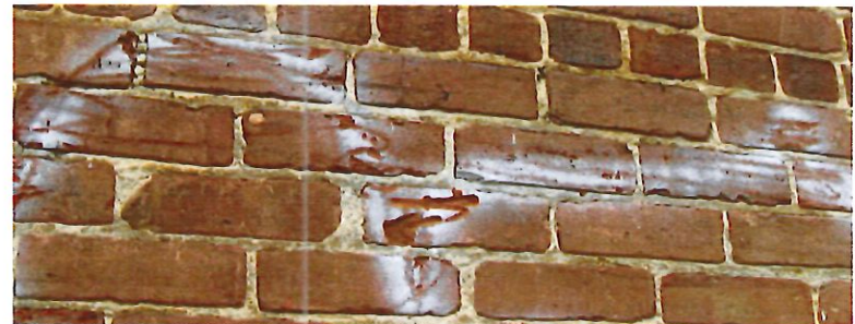
Example of irreversible damage to brick caused by high-pressure washing in an unsuccessful attempt to remove graffiti. (Photo from Easements Atlanta.)
