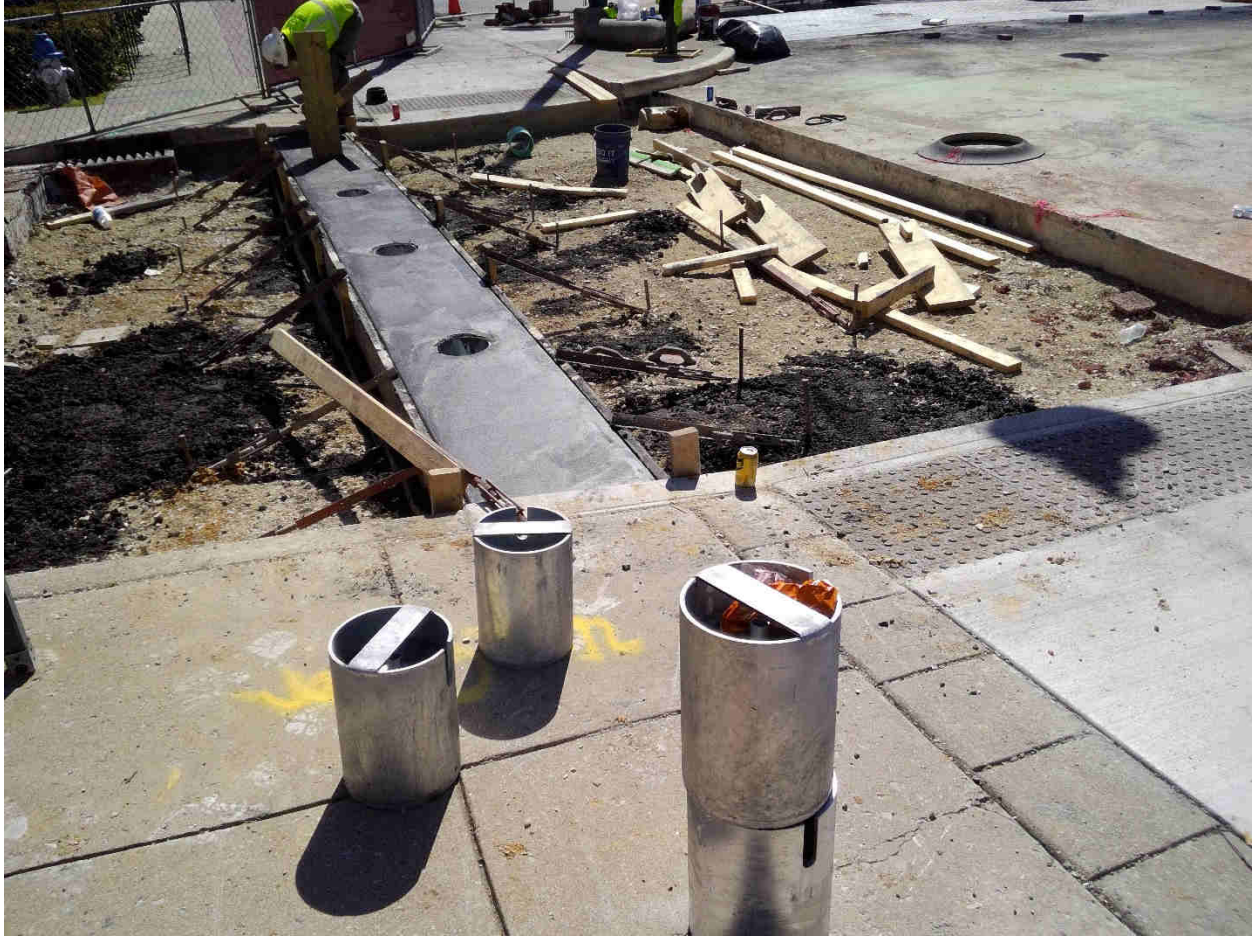
Bollard footer at North leg Grant St. Intersection. Upside down bollard anchors staged on sidewalk.
