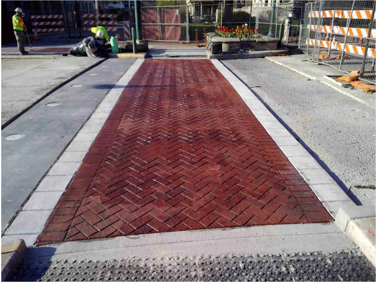
Crosswalk at South leg Grant St. Intersection, complete. Shown here with sealer drying.
