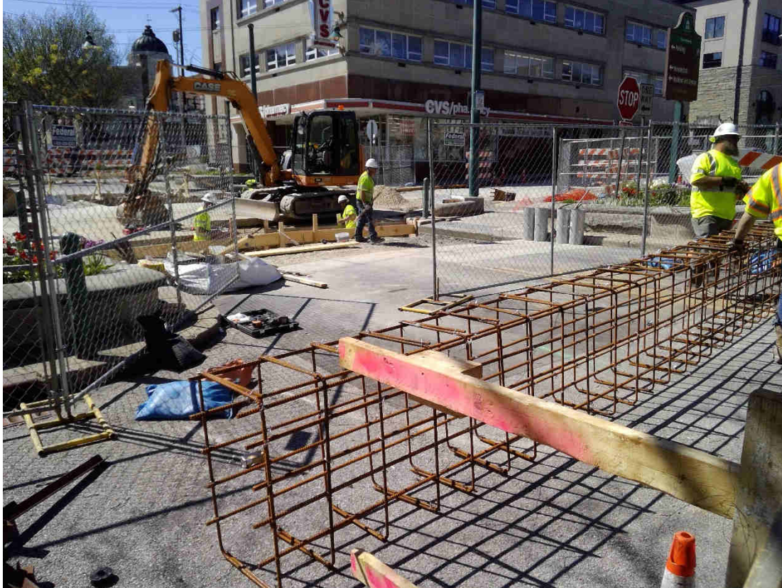
East leg Grant St. re-bar basket for bollard footer before it is set in the excavated hole. The West bollard footer in the foreground is being constructed.
