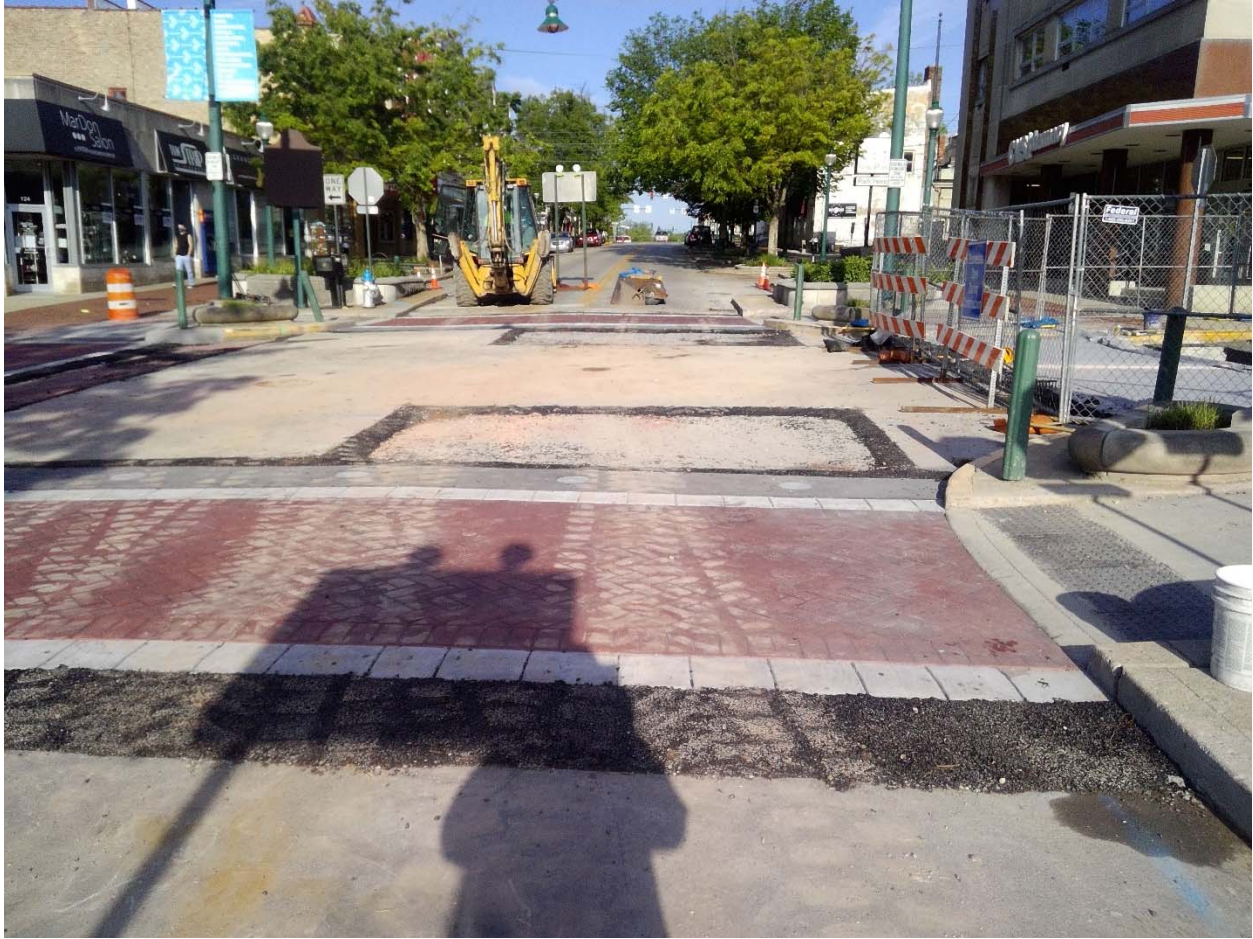
Opened up 3 legs, Washington St., Intersection on Wednesday. North leg left closed while the concrete cures until Monday, 5/11.
