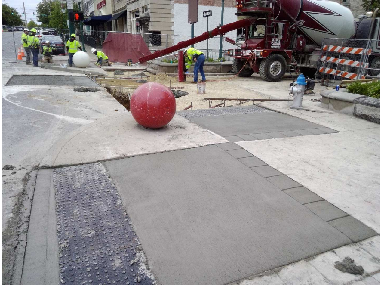
Walnut St., East leg new ADA compliant curb ramps are all in.
