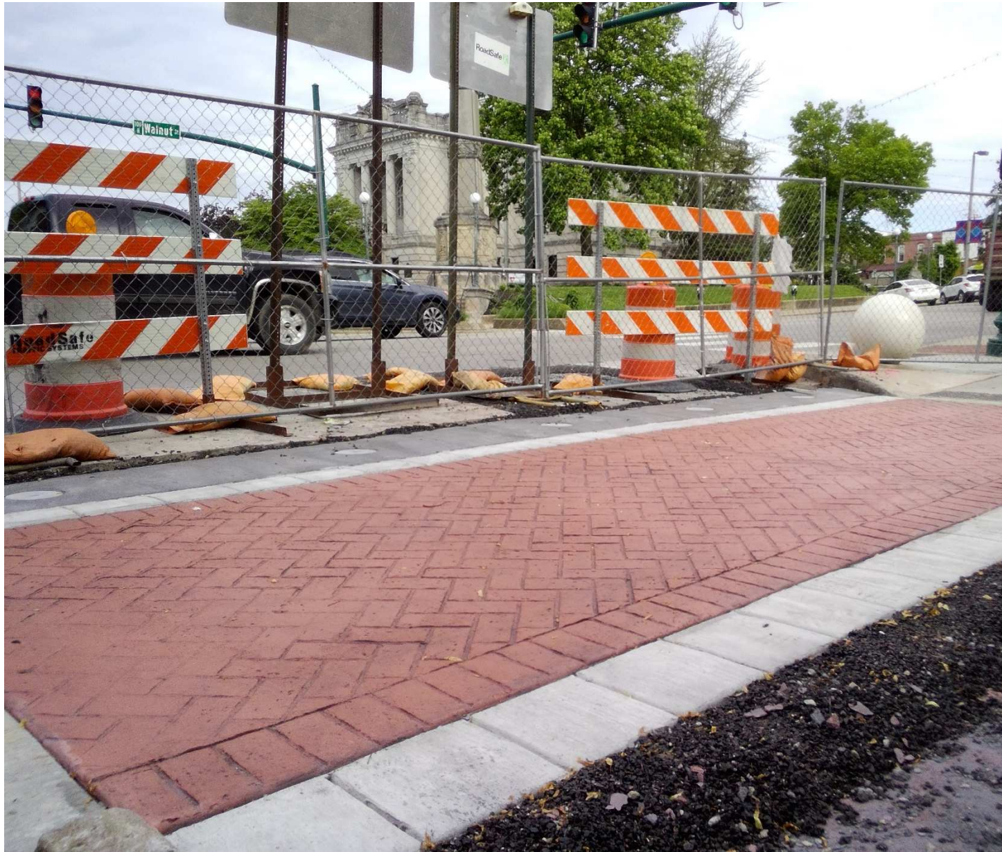
East leg, Walnut St., crosswalk and ADA compliant curb ramps finished and bollard footer array installed.
