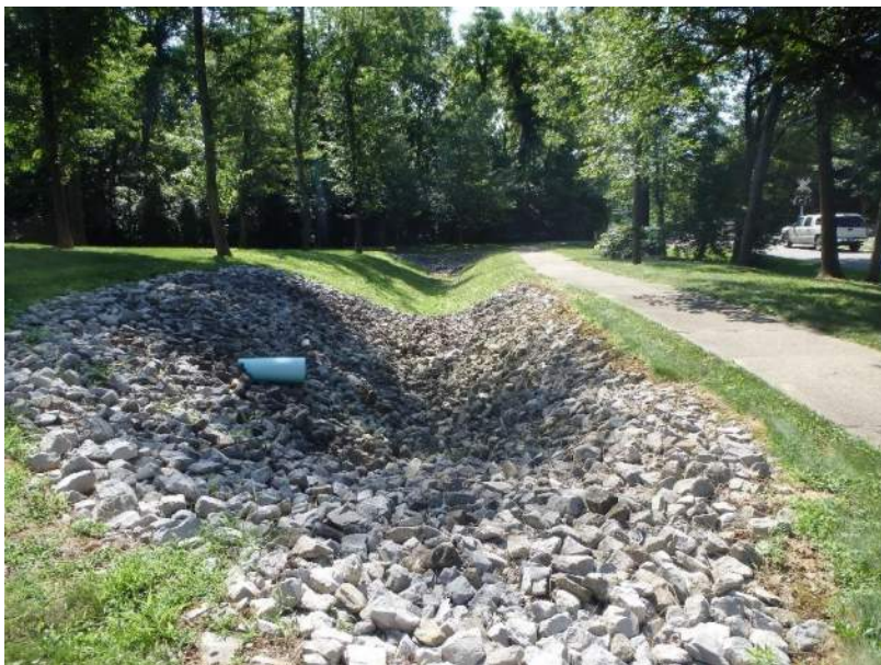
PP5 – Private property stormwater management feature
