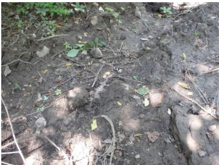
PP6 –Buried drop inlet
