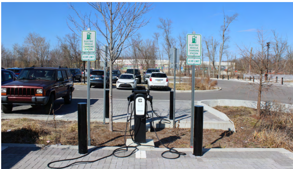
EV charging stations at Switchyard Park
