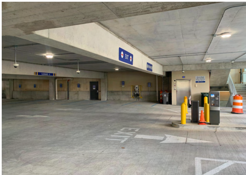
Other City LED Lighting Projects, LED lighting in Trades District Garage
