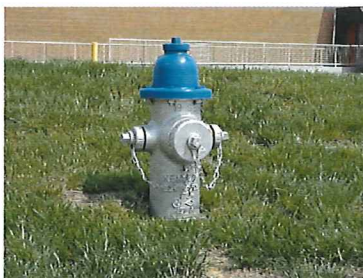
Aluminized Hydrant Barrel City of Bloomington Utilities Owned and Maintained
