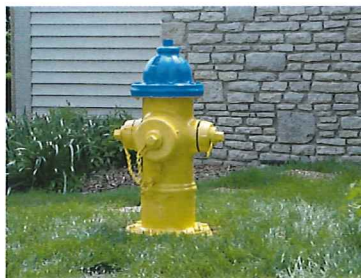
Yellow Hydrant Barrel Private Owned and Maintained
