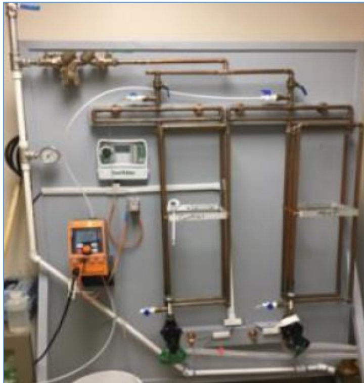
Example of a pipe loop study set-up.
