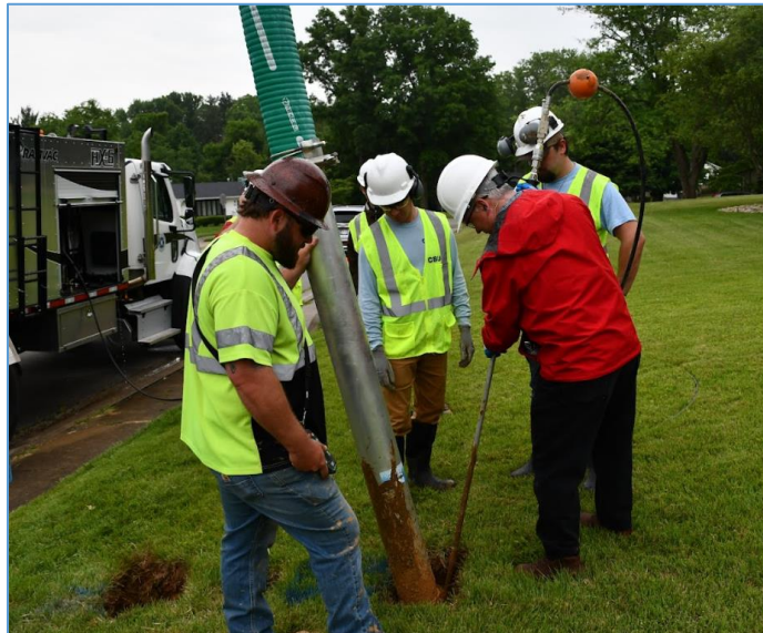
Pot-holing on both sides of the water meter pit.
